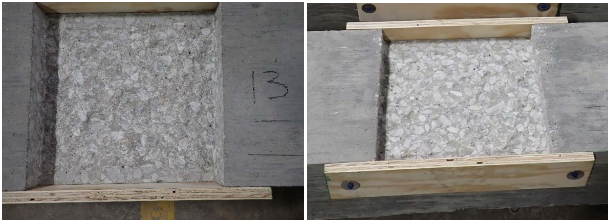
Figure 3. No anchor in 1-1/2-inch cavity
