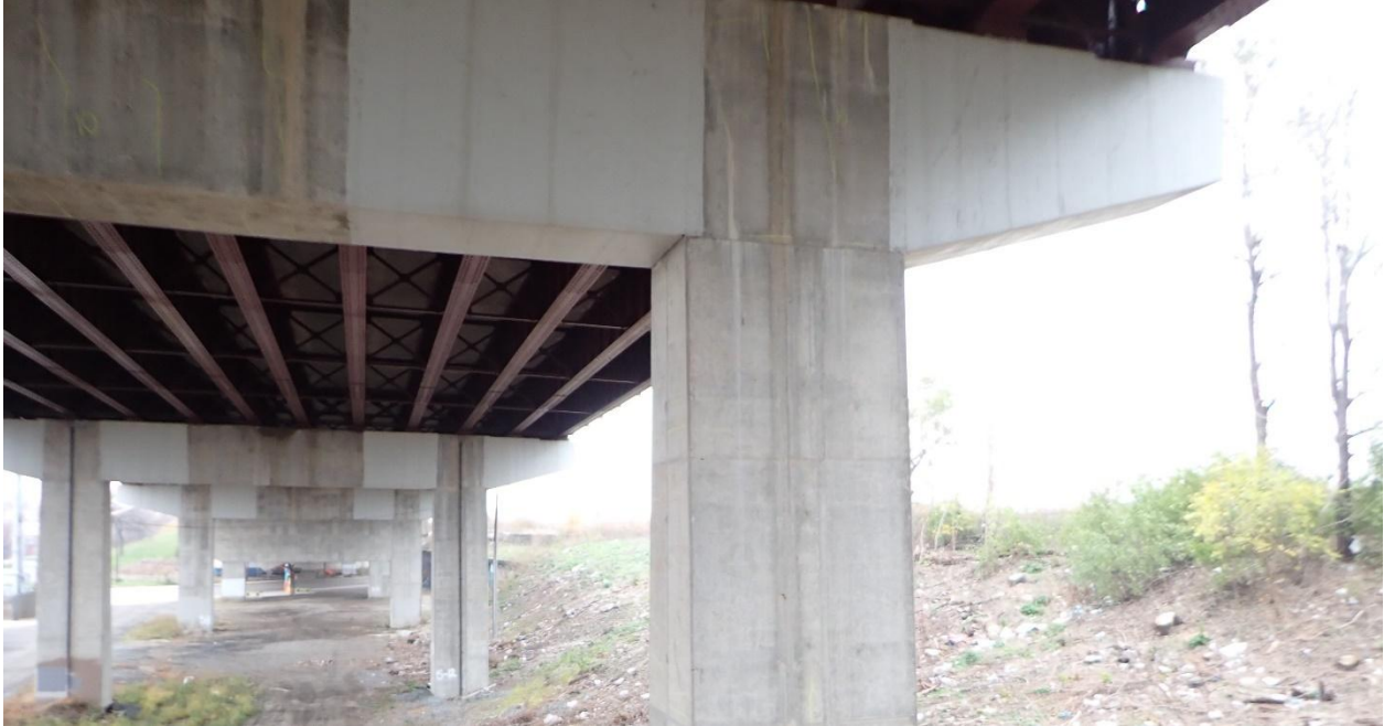
Figure A.4. FRP repairs (painted in white) wrapped around pier caps. (These were structural repairs and extend further than necessarily required for VOH repairs.)
