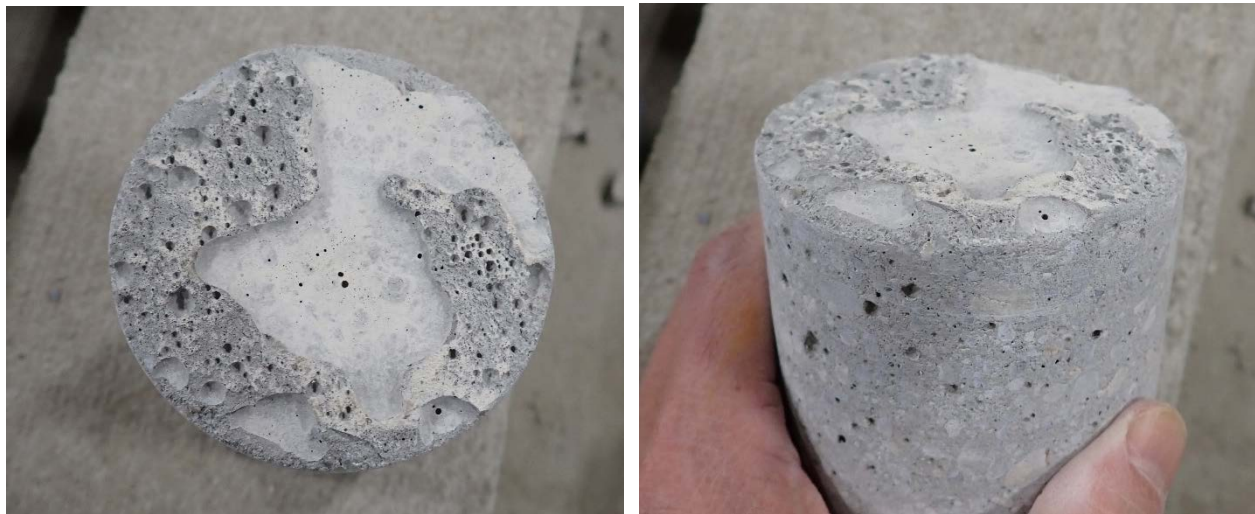
Figure 17. Pull-off test sample for an overhead, form-and-pour repair (Material F2); sample separated during coring at the interface where large air voids in the material were present.
