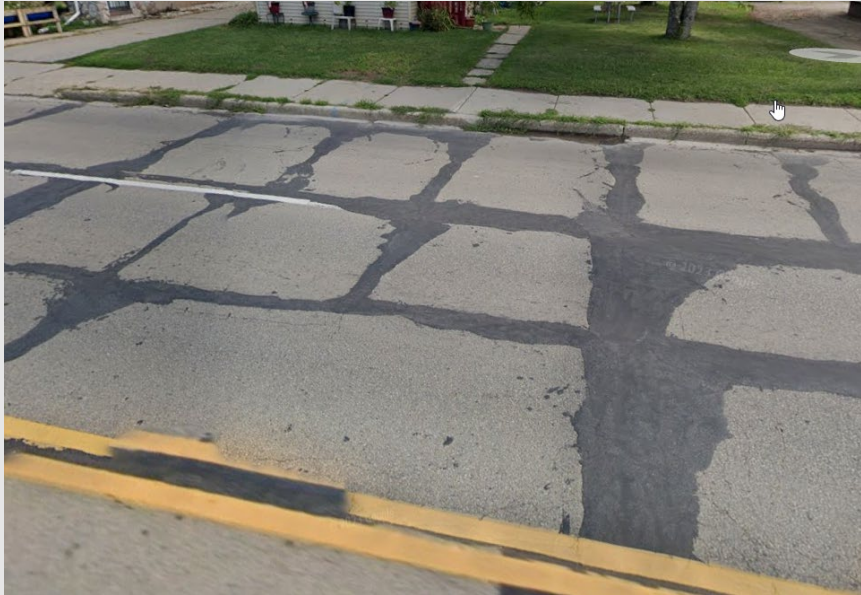
Pavement Deterioration/Ride Quality
