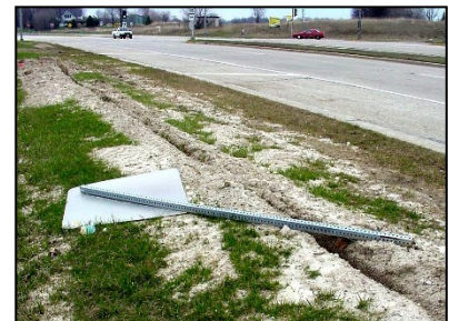
Figure 1: Improper Sign Removal
