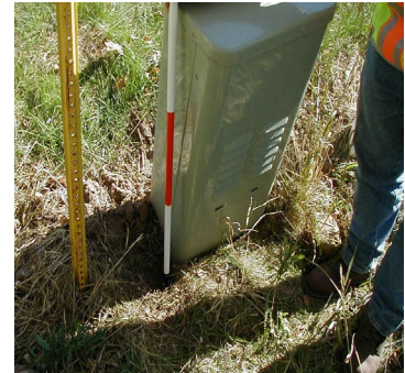
Figure 1. Pedestal too close to ROW pin.
