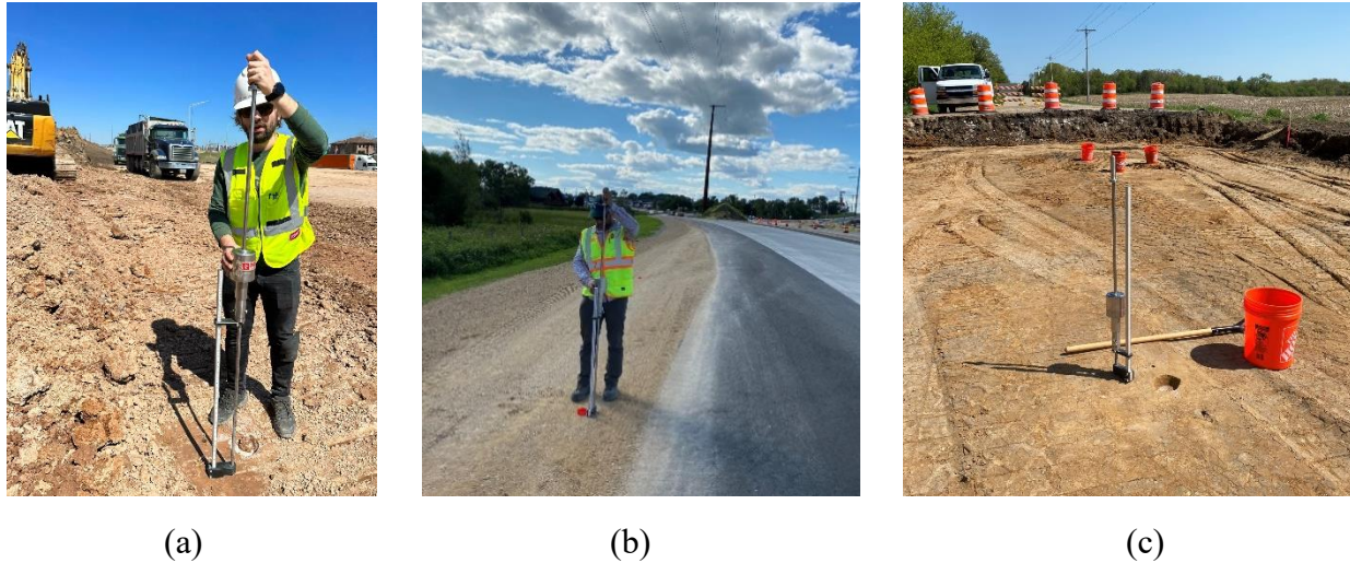
Figure 3.7 Dynamic cone penetrometer (DCP) test performed at (a) Milwaukee County, (b) Juneau County and (c) Racine County
