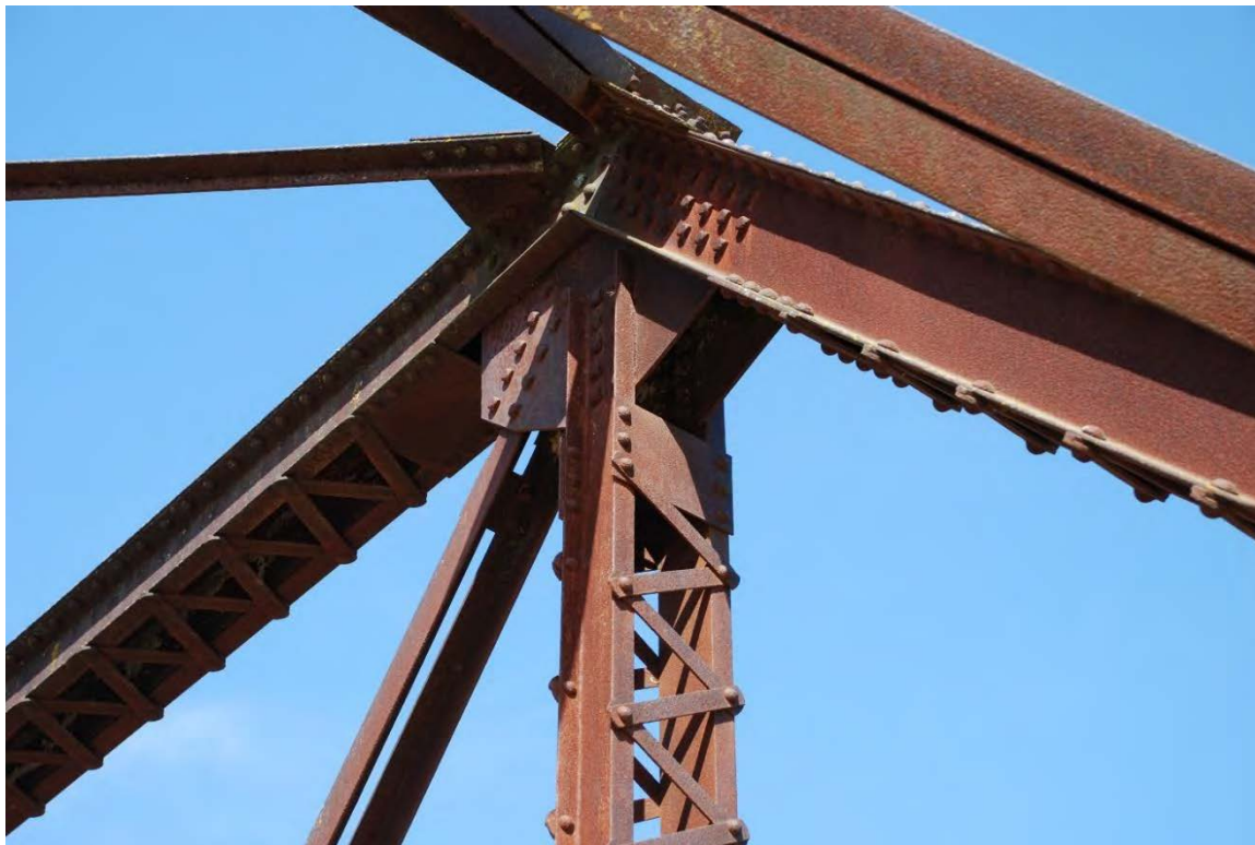
Figure 10. Riveted connection showing details of top chord, vertical, and diagonals members, view facing north.
