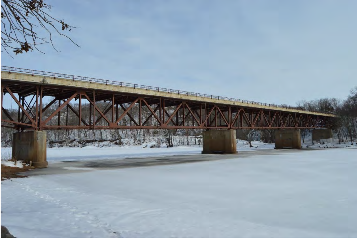
B-48-0224, looking NE
