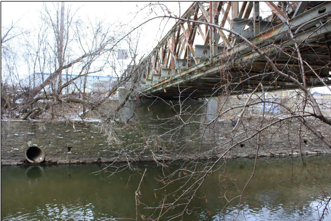
P-40-0658, Concrete abutment and stone retaining wall, facing north across Menomonee River.
