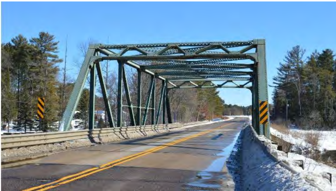
Figure 12. Photographs of two truss bridges: a 99-foot-long standard-plan 1917 Pratt thru truss with a 16-foot-wide deck (top) and a 104.7-foot-long standard-plan 1936 Pratt thru truss with a 31-foot-wide deck (bottom). Notice the wider, larger, solid steel truss members in the 1936 bridge and the limited weight capacity sign adjacent to the 1917 truss. Later truss bridges were made to carry much heavier loads.
