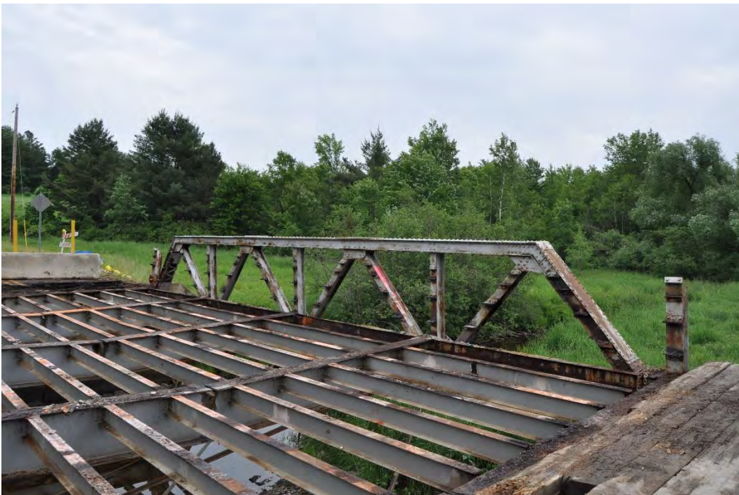
Stettin Drive Bridge (P-37-0203), interior of south truss and view of the floor beams, decking and railing removed, looking southeast.
