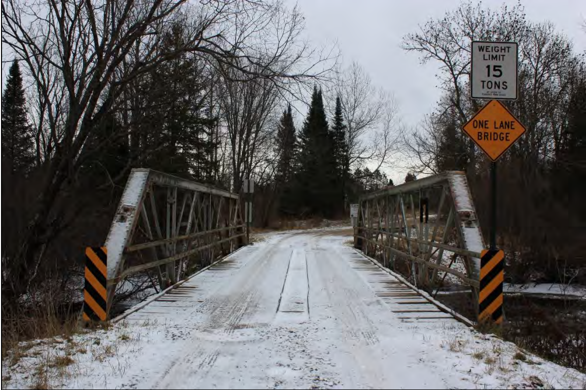
P-19-0013, Overview of bridge setting, deck, and approach, facing east on Pentoga Road toward the Michigan border.
