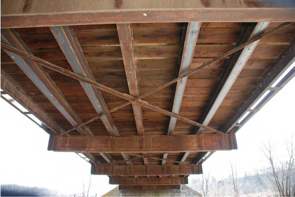
Figure 18. Early standard plan wood deck (view from below) on the Richardson Bridge (AHI No. 245600, P-33-0213), 1917.
