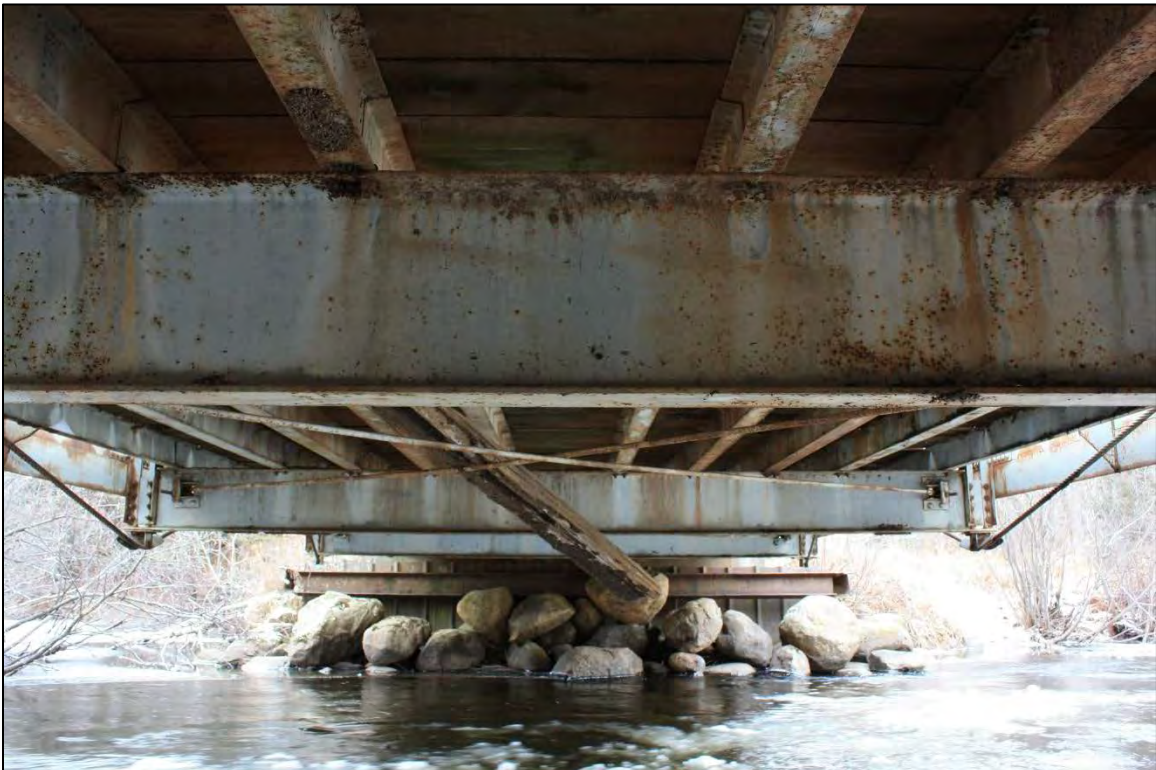
P-19-0013, Superstructure underside toward concrete abutment and sheet metal and I-beam crib, facing east across Brule River.
