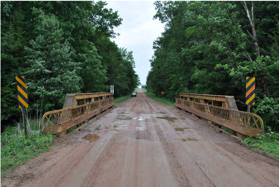
Photo 4 of 4: Rosedale Avenue Bridge (P-37-0179), north approach, looking south along Rosedale Avenue.
