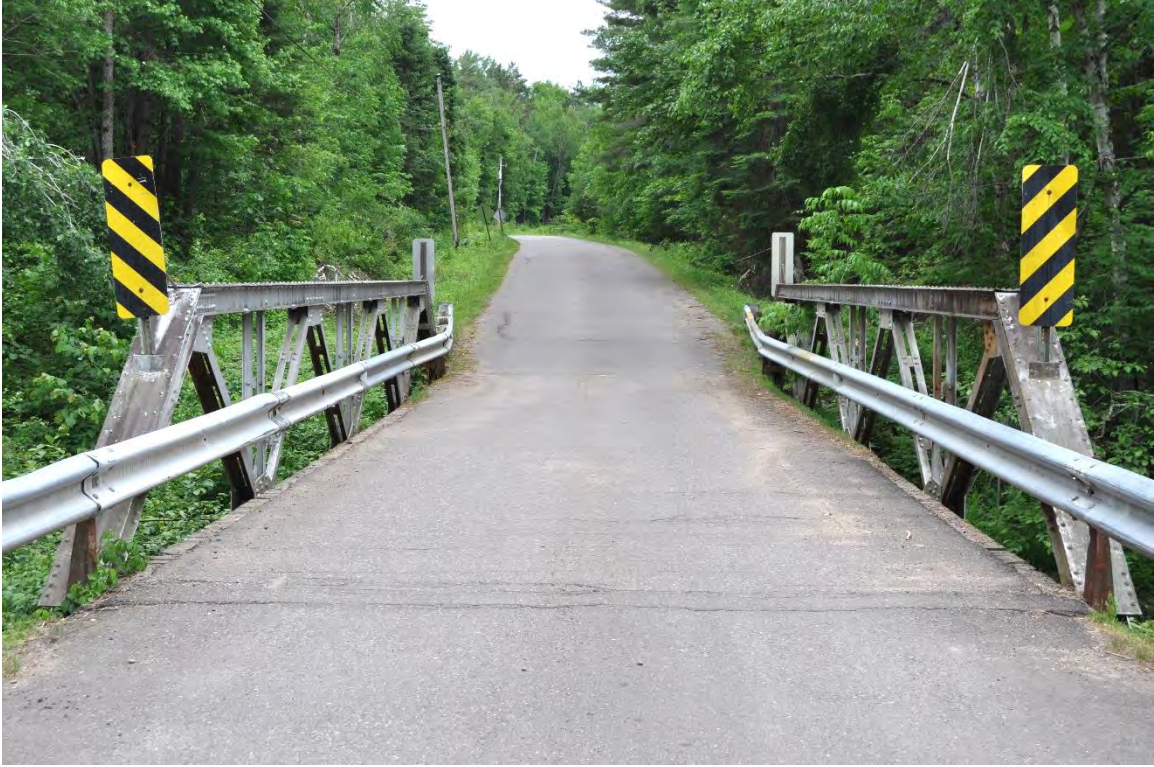
Figure 20. Addition of modern guardrail on the Josie Creek Road Bridge (AHI No. 245702, P-54-0906), 1915.
