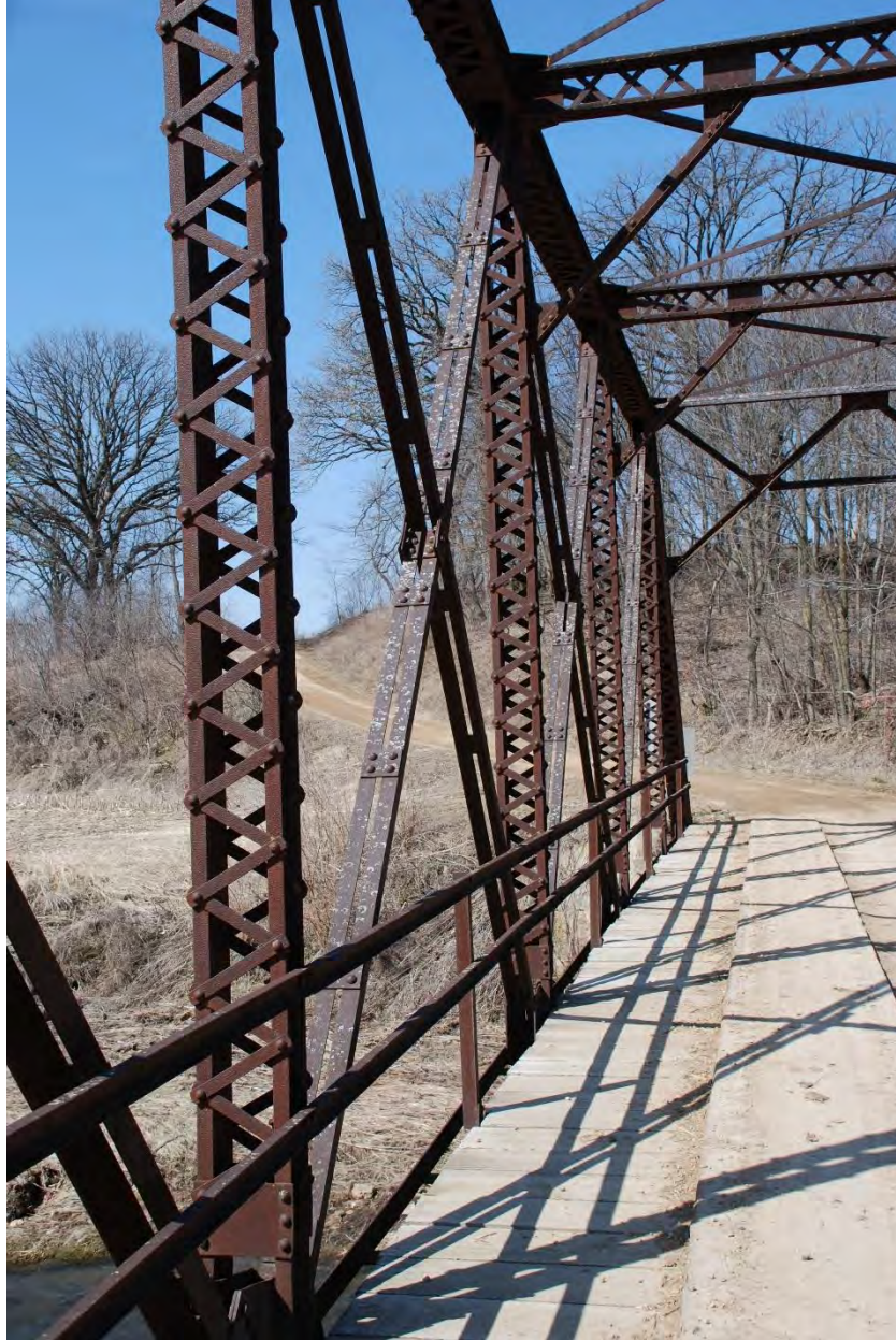
Figure 9. Vertical and diagonals members, and railing, view facing west. This photo shows the two lines of channel railing, two channel verticals, and two angle diagonals.
