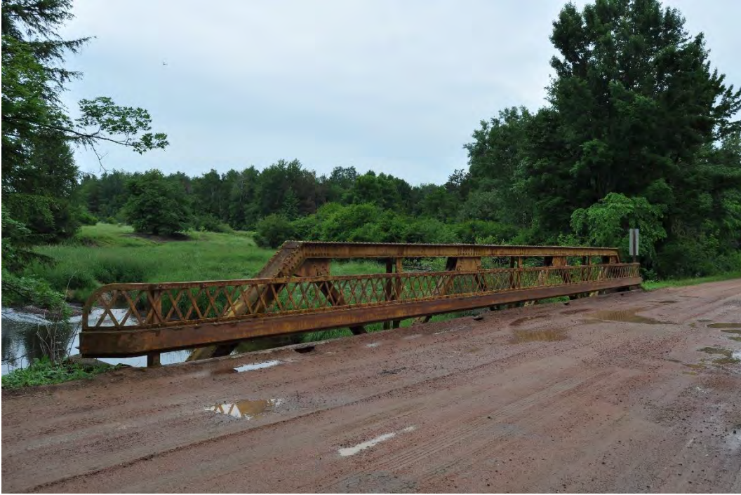
Photo 3 of 4: Rosedale Avenue Bridge (P-37-0179), interior of west elevation, viewed from south end of the bridge, looking northwest.
