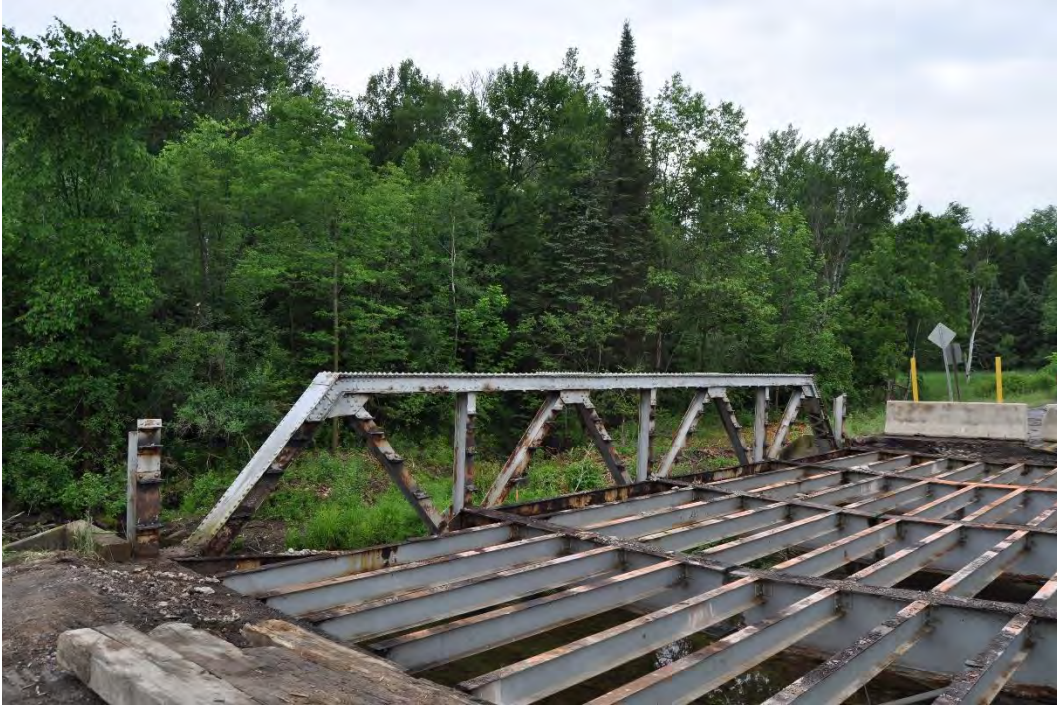
Stettin Drive Bridge (P-37-0203), interior of north truss and view of the floor beams, decking and railing removed, looking northwest.
