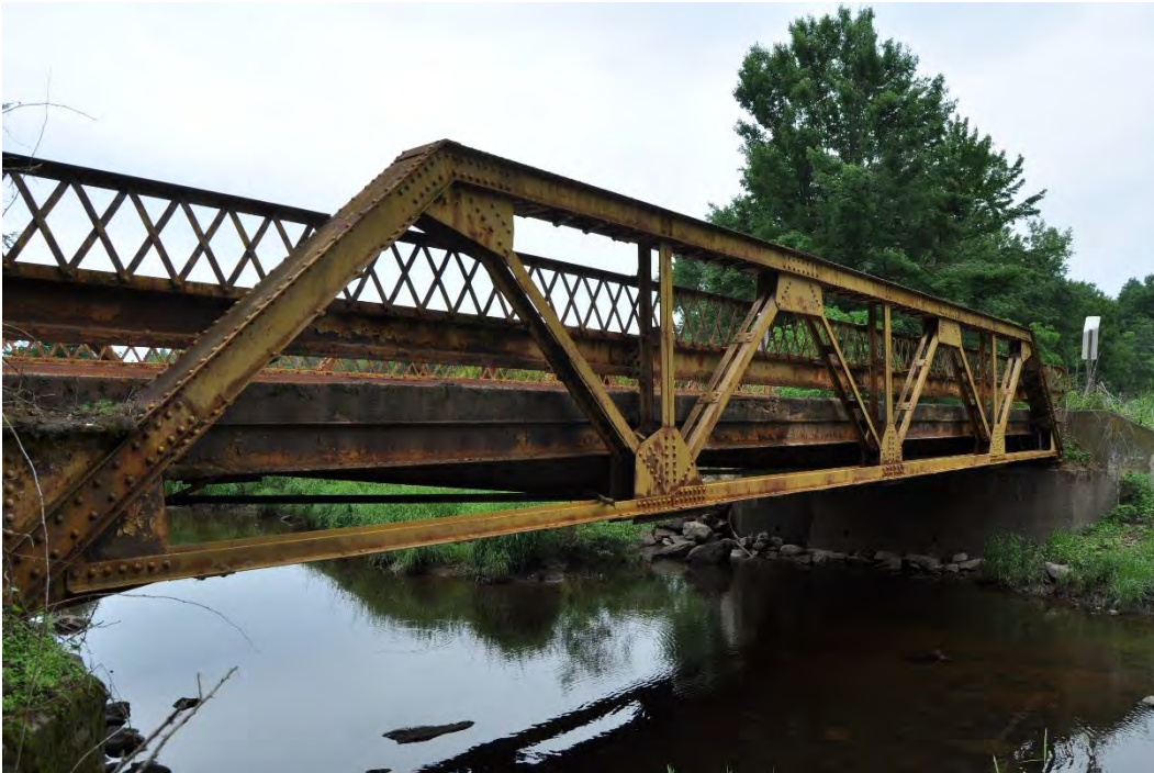
Photo 2 of 4: Rosedale Avenue Bridge (P-37-0179), east elevation, viewed from south bank of Big Eau Pleine River, looking northwest.
