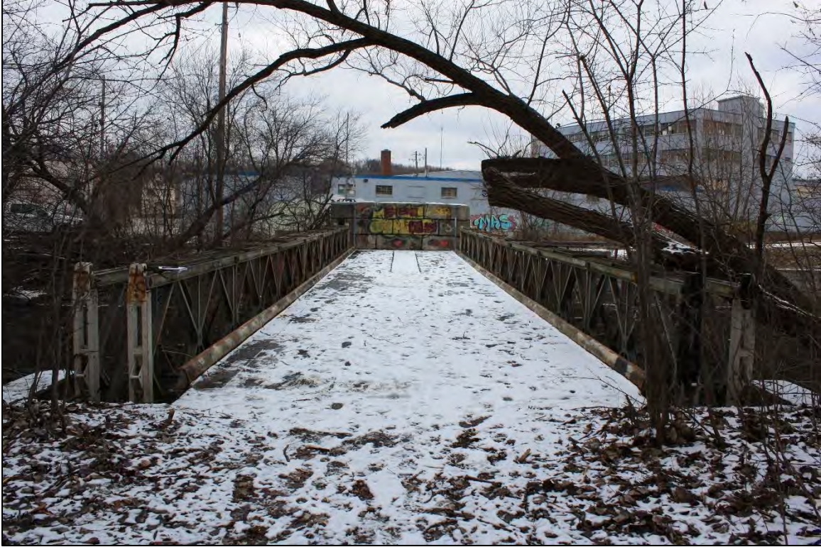
P-40-0658, Overview of bridge setting, deck, and approach, facing north from Doyne Park.
