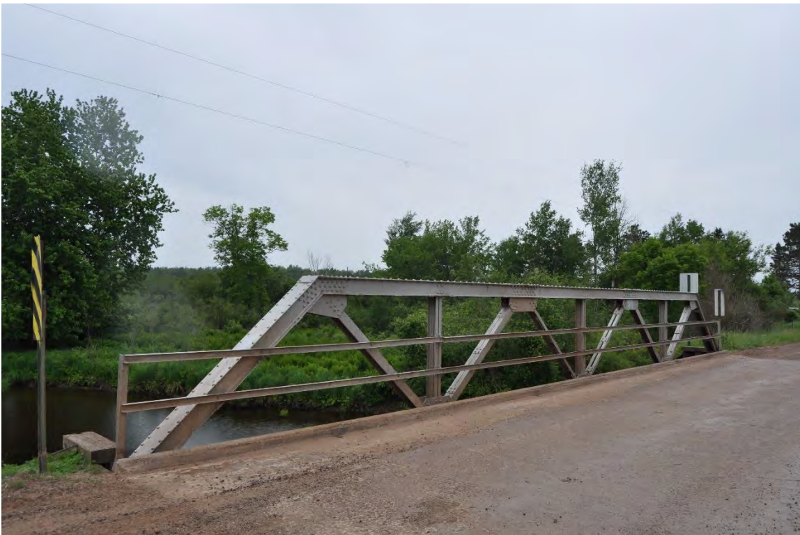
Photo 4 of 4. P-50-0091, interior of east truss and overview of decking, looking southeast.
