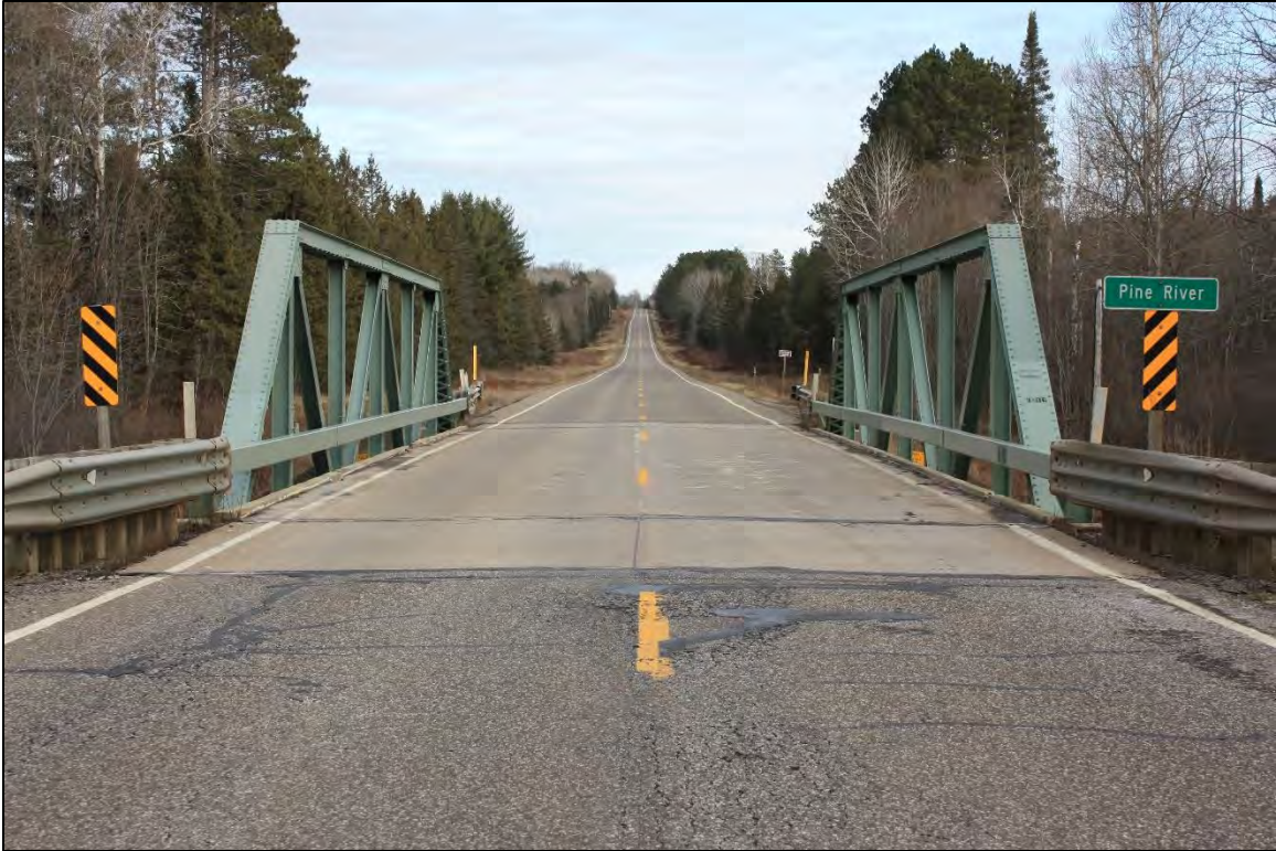
B-19-509, Overview of bridge setting, deck, and approach, facing west on STH 101.
