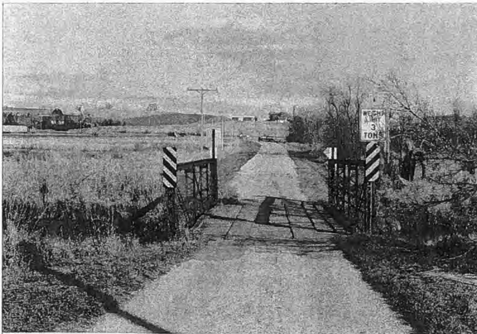
Beaver Dam Road Bridge (P-66-055), Town of Addison, Washington County Top: South elevation - Source: J.A. Hess, 1986 Bottom: Approach - Source: J.A. Hess, 1986
