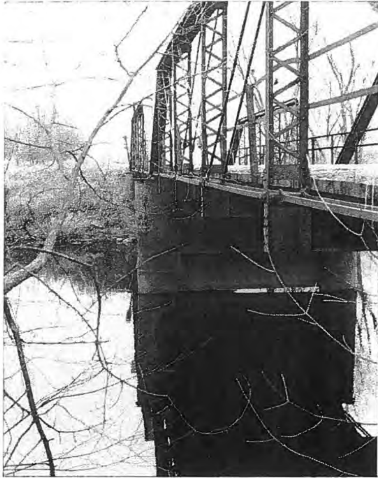
Sawyer Avenue Bridge (P-60-125), Town of Hammel, Taylor County Bottom chord, northeast elevation - Source: J.A. Hess, 1986
