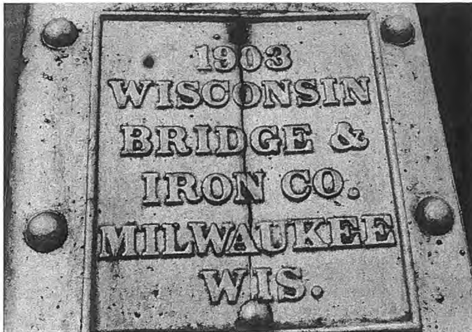
Nachtway Road Bridge (P-36-088), Town of Gibson, Manitowoc County Top: East elevation - Source: J.A. Hess, 1986 Bottom: Detail of builder's plate - Source: J.A. Hess, 1986
