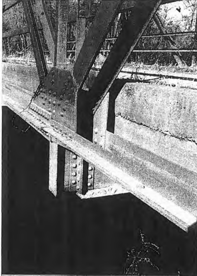
Willenberg Bridge (P-62-320), Town of Genoa, Vernon County Detail of bottom chord and hanger - Source: J.A. Hess, 1986
