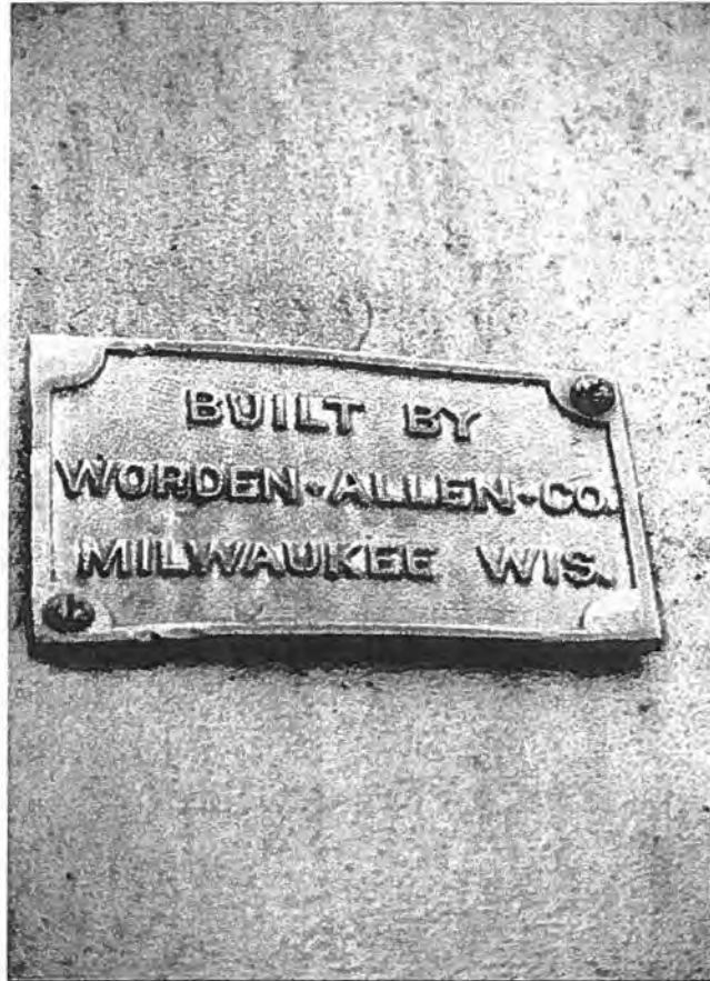
Heath Bridge (P-57-068), Town of Weirgor, Sawyer County Detail of bridge plate on inclined endpost, southeast end - Source: J.A. Hess, 1986
