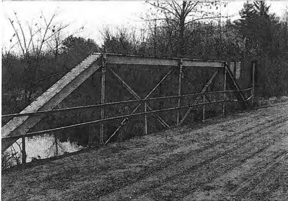
Mulberry Lane Bridge (P-60-117), Town of Medford, Taylor County South side of north elevation - Source: J.A. Hess, 1986
