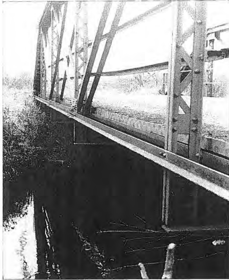
Larson Road Bridge (P-54-107), Town of Grant, Rusk County Detail of north side of south elevation - Source: J.A. Hess, 1986
