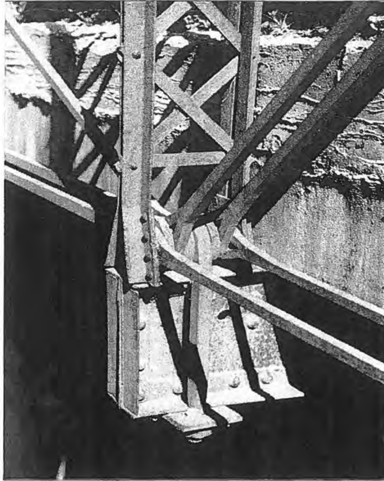
Bear Creek Bridge (P-52-224), Town of Buena Vista, Richland County Detail of pin connection - Source: Wisconsin Department of Transportation, 1981
