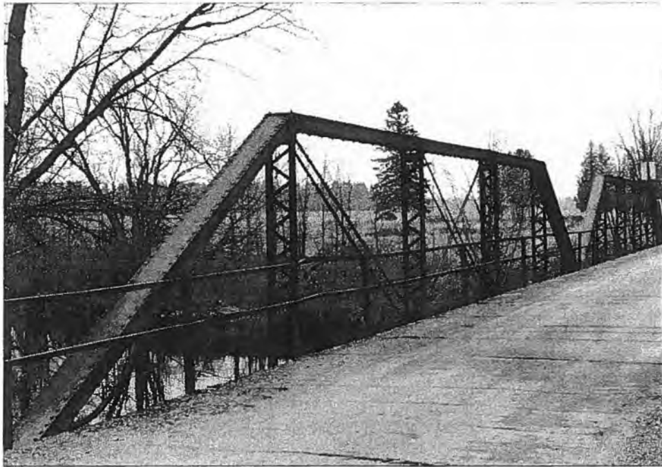
Sawyer Avenue Bridge (P-60-125), Town of Hammel, Taylor County Southwest side of northeast elevation - Source: J.A. Hess, 1986
