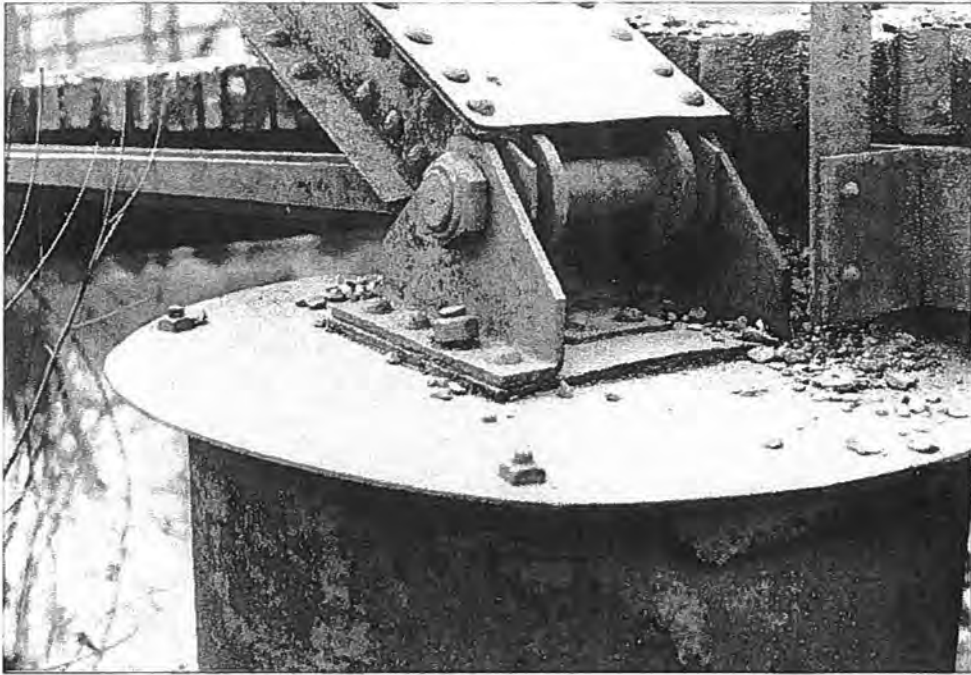
Sawyer Avenue Bridge (P-60-125), Town of Hammel, Taylor County Detail of bearing, south end - Source: J.A. Hess, 1986
