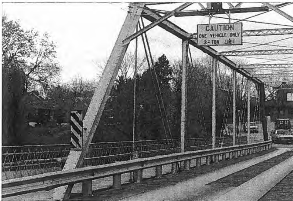
Bridge Street Bridge (P-45-700), Village of Grafton, Ozaukee County Top: North elevation - Source: J.A. Hess, 1986 Bottom: North elevation, south side - Source: J.A. Hess, 1986
