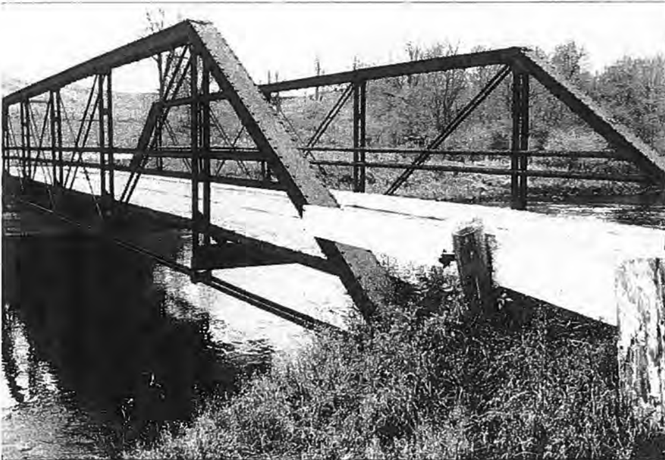
Blomberg Road Bridge (P-58-111), Town of Grant, Shawano County Top: West elevation - Source: J.A. Hess, 1986 Bottom: South approach - Source: J.A. Hess, 1986
