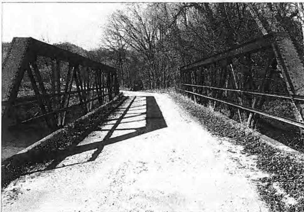
Willenberg Bridge (P-62-320), Town of Genoa, Vernon County Top: West elevation - Source: J.A. Hess, 1986 Bottom: Approach - Source: J.A. Hess, 1986
