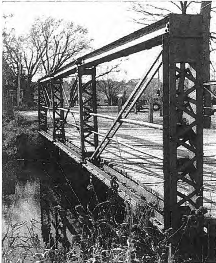
Allenton Park Bridge, Town of Addison, Washington County South elevation - Source: J.A. Hess, 1986
