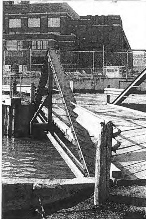
Sauk Creek Bridge (P-45-714) City of Port Washington, Ozaukee County East elevation - Source: J.A. Hess, 1986
