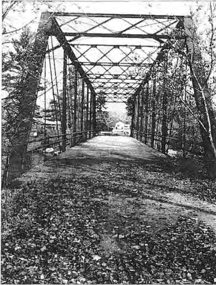
Van Laenen Road Bridge (P-42-081), Town of Stiles, Oconto County South approach - Source: J.A. Hess, 1986
