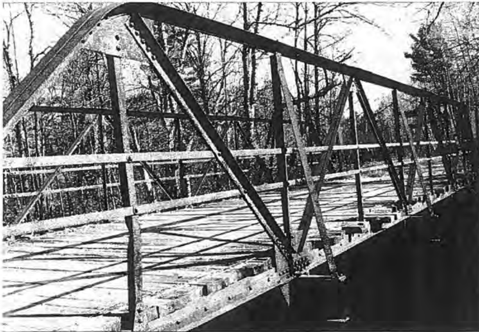
Iron Bridge Road Bridge (P-42-901), Town of Armstrong, Oconto County Top: South elevation - Source: J.A. Hess, 1986 Bottom: Detail of south elevation - Source: J.A. Hess, 1986
