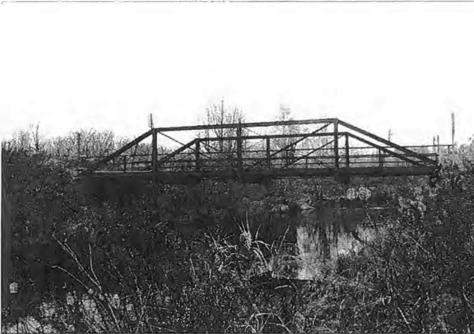
Broken Arrow Road Bridge (P-54-125), Town of Willard, Rusk County South elevation - Source: J.A. Hess, 1986
