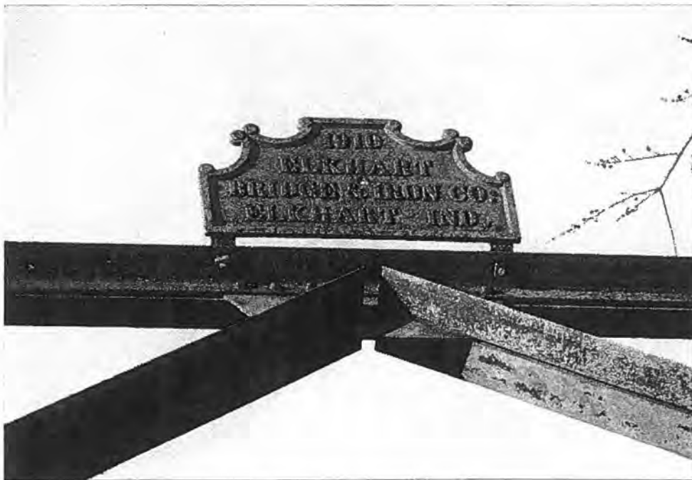
Ferndale Road Bridge (P-38-096), Towns of Lake and Grover, Marinette County Top: South approach - Source: J.A. Hess, 1986 Bottom: Detail of builder's plate - Source: J.A. Hess, 1986
