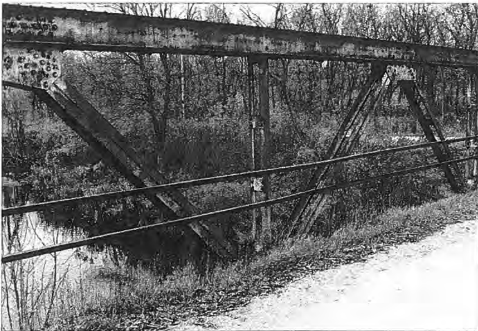
Melnik Road Bridge (P-36-089), Town of Gibson, Manitowoc County Top: West elevation - Source: J.A. Hess, 1986 Bottom: West truss, east elevation - Source: J.A. Hess, 1986
