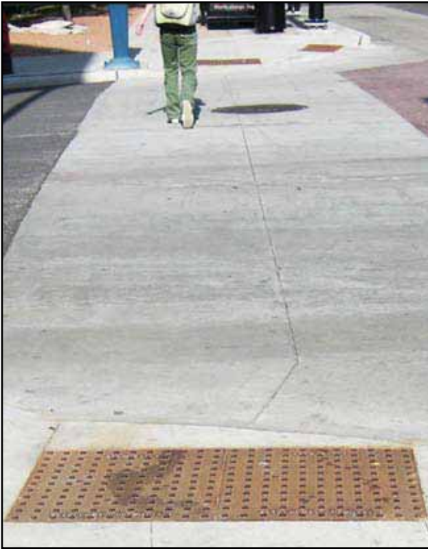
Exhibit 5-50: The curb ramp is perpendicular to the roadway with a minimized triangle between detectable warnings and crosswalk.
