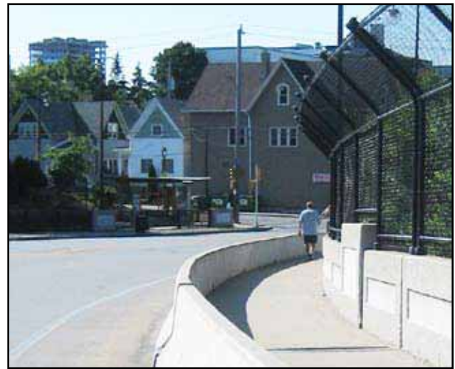
Exhibit 5-76: On bridges with higher speeds, substantial traffic volume or significant curvature, it may be necessary to include a jersey barrier between the walking area and the roadway.
