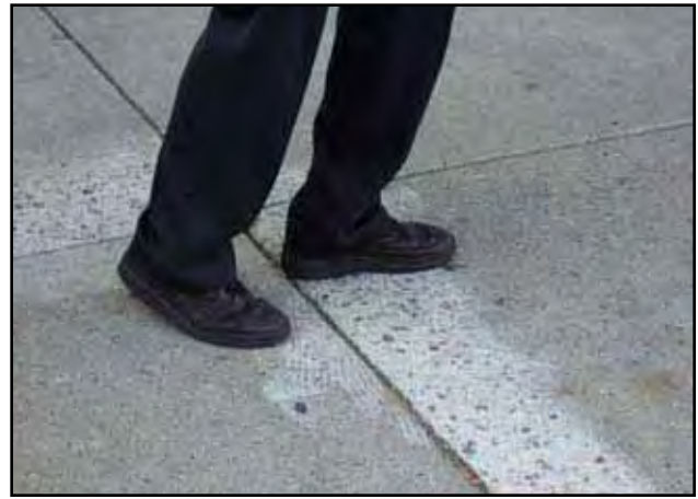
Exhibit 5-28: Changes in level can create tripping hazards. Any changes in level between \frac{1}{4} and \frac{1}{2} inch should be beveled.
