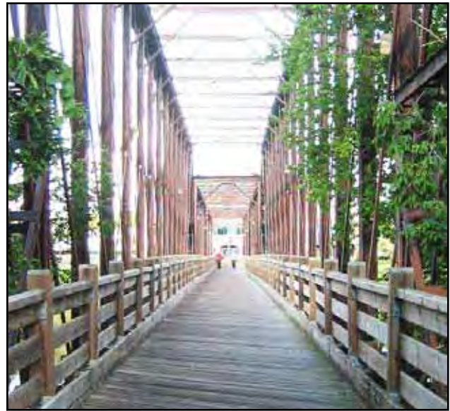
Exhibit 5-1: Where a river bisects a community, a bridge can help to mitigate the barrier effect on pedestrians.
