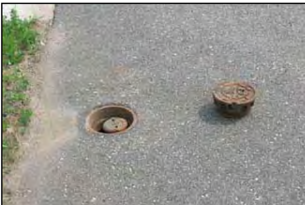
Exhibit 5-32: Maintenance features can instead be encircled by a frost sleeve to prevent frost heaving.
