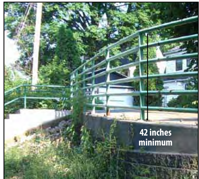
Exhibit 5-90: A protective edge along a trail must have a minimum height of 42 inches.
