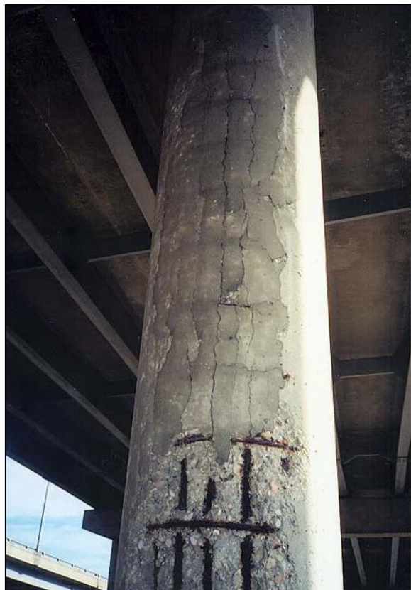
Figure 2.5.3.1-6: Delaminated and Spalled Column - Condition State 3
