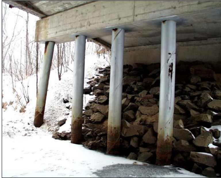
Figure 2.5.2.4-1: Heavy Corrosion at the Ground Line on Painted Steel Piles - Condition State 4
