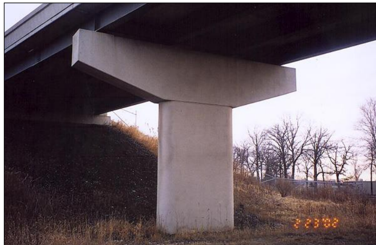
Figure 2.5.3.1-2: Hammerhead Pier Reinforced Concrete Column – Condition State 1 (The cap of the hammerhead pier is reported under Element 234).
