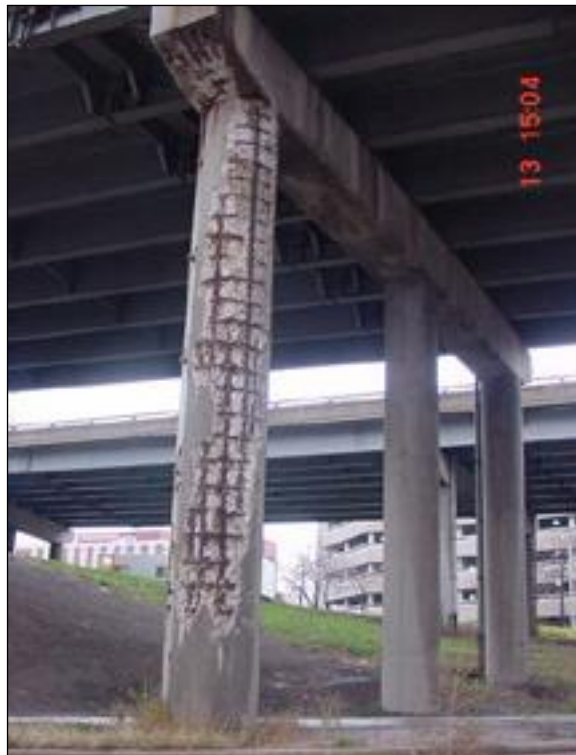
Figure 2.5.3.1-8: Heavily Spalled Column - Condition State 4
