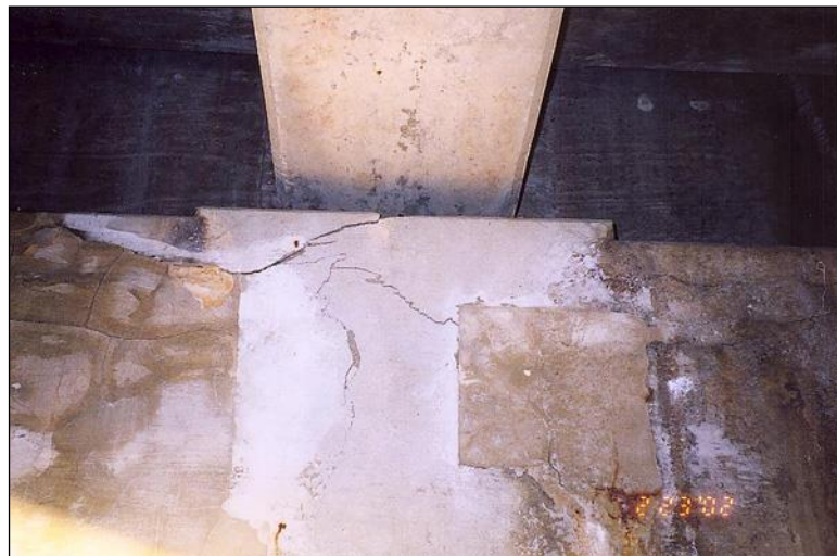
Figure 2.5.3.3-5: Abutment Delaminations Under the Bearing – Condition State 2
