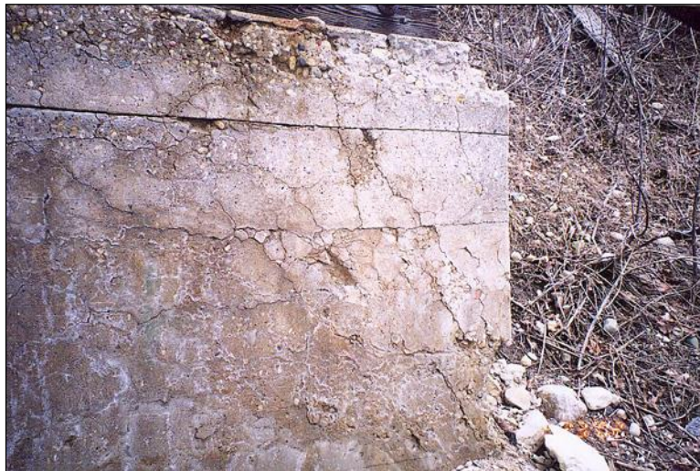
Figure 2.5.3.2-2: Cracked, Delaminating and Spalled Reinforced Concrete Pier Wall – Condition State 3
