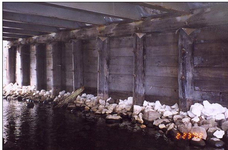
Figure 2.5.5.4-1: Timber Abutment, Pier Cap, and piles - Condition State 2
