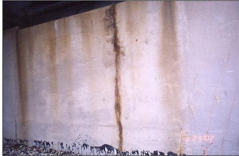
Figure 2.5.3.3-4: Vertical Crack in an Abutment – Condition State 2
