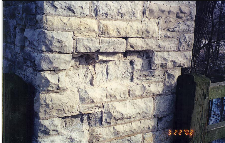
Figure 2.5.6.2-4: Split and Spalled Masonry Units – Condition State 3
