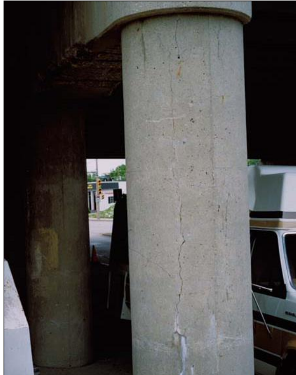
Figure 2.5.3.1-3: Concrete Column with Vertical Crack - Condition State 2
