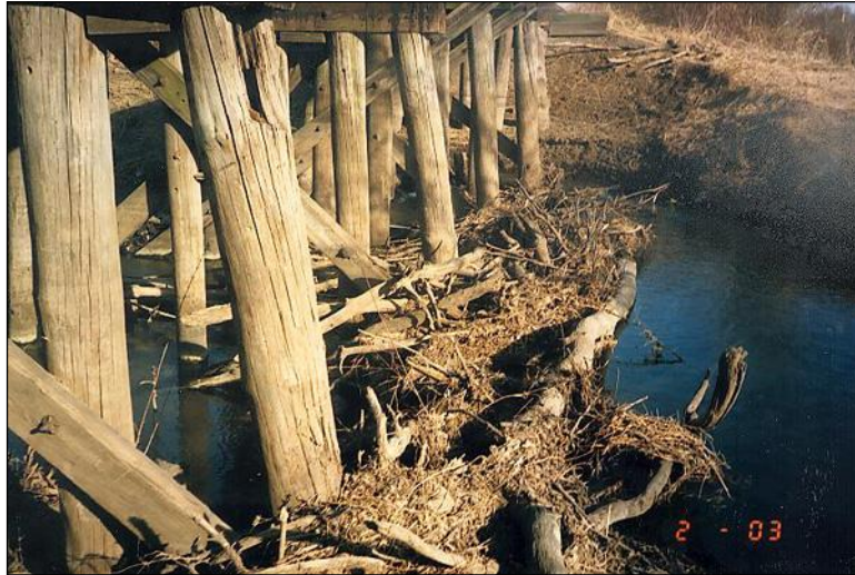
Figure 2.5.5.5-1: Timber Piling – Most in Condition State 2
