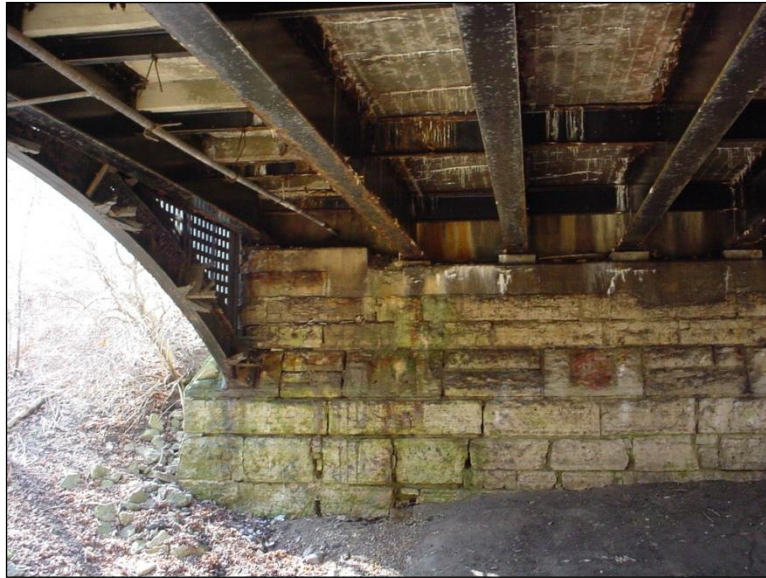
Figure 2.5.6.2-2: Masonry Abutment with Moderate Mortar Deterioration – Condition State 2
