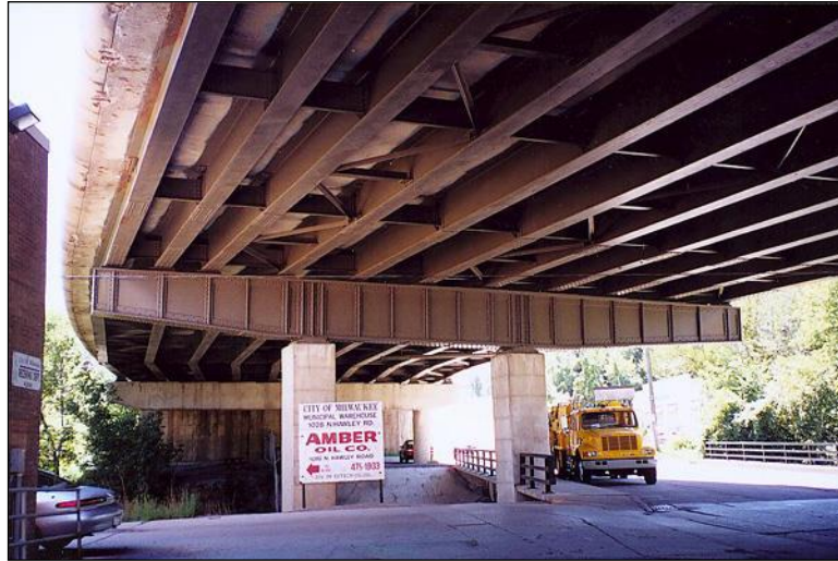
Figure 2.5.2.6-1: NSTM Riveted Steel Box Girder Pier Cap. Note that the superstructure girders bear on the pier cap's top flange by way of bearing devices
