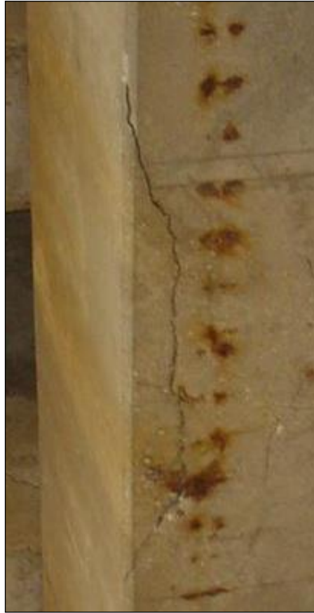
Figure 2.5.3.6-4: Delaminations on the Underside of a Pier Cap - Condition State 2
