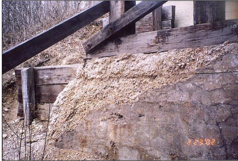
Figure 2.5.3.2-3: Disintegration of a Reinforced Concrete Pier Wall – Condition State 3
