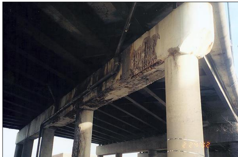
Figure 2.5.3.6-5: Pier Cap with Widespread Spalling – Condition State 3
