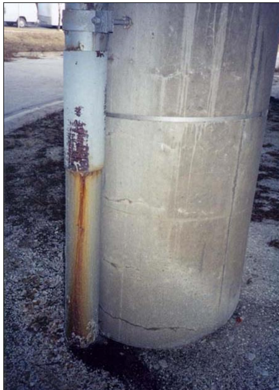
Figure 2.5.3.1-4: Transverse Flexural Cracks at the Base of a Column - Condition State 2
