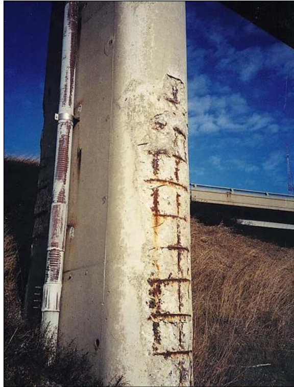
Figure 2.5.3.1-7: Spalling on a Reinforced Concrete Shaft - Condition State 3
