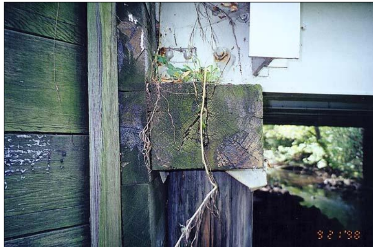
Figure 2.5.5.6-2: Split Pier Cap End (Note Plant Growth) - Condition State 3
