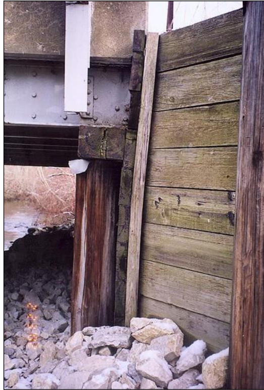
Figure 2.5.5.4-2: Bulging of a Timber Abutment (Settlement Defect) – Condition State 2
