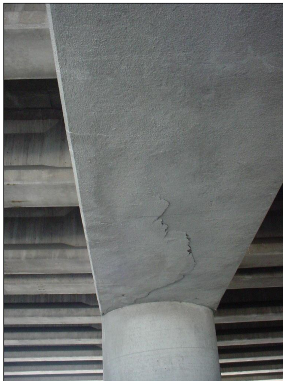
Figure 2.5.3.6-3: Delamination on the Underside of a Pier Cap – Condition State 2
