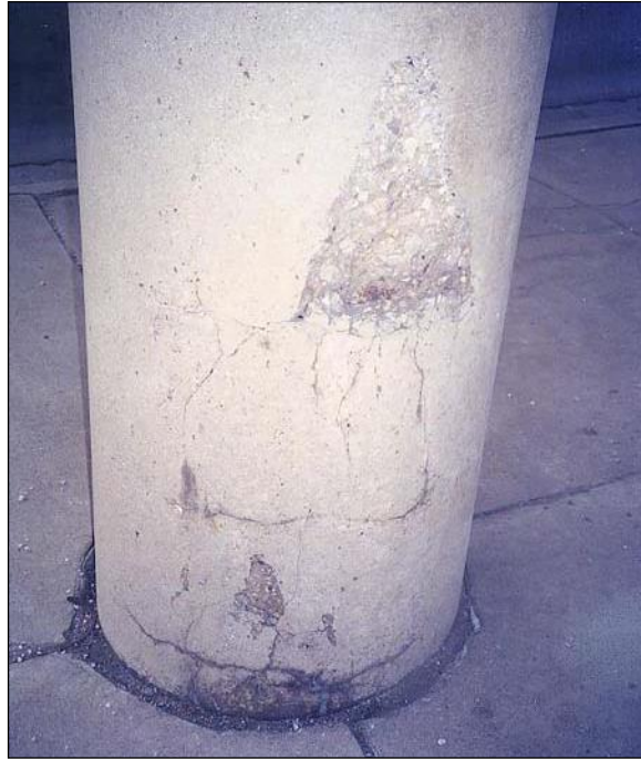
Figure 2.5.3.1-5: Column Spall with No Exposed Rebar - Condition State 2
