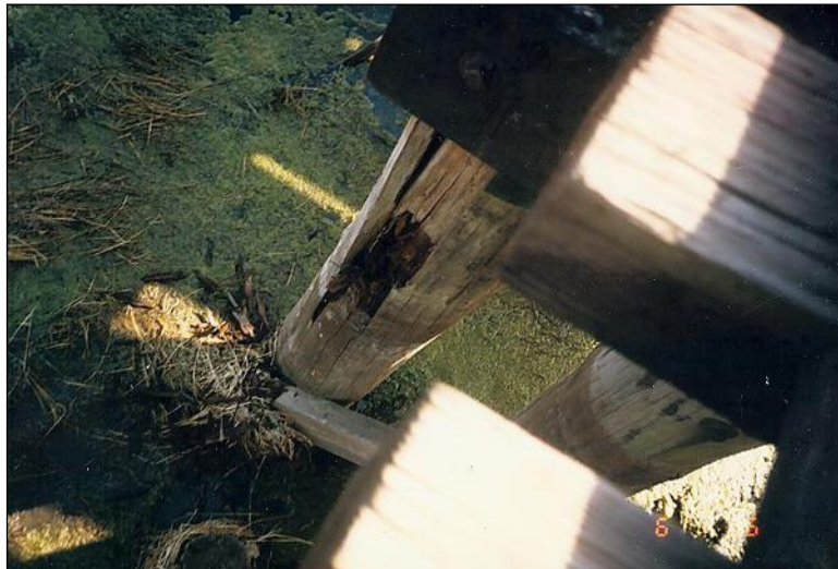
Figure 2.5.5.5-2: Split and Decayed Timber Piling- Condition State 3
