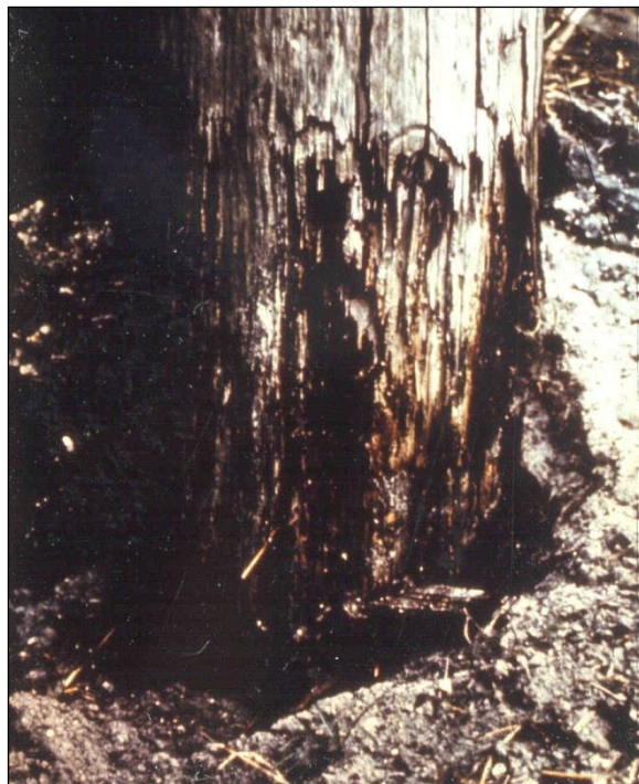
Figure 2.5.5.5-4: Timber Pile Decay at Ground Line – Condition State 3
