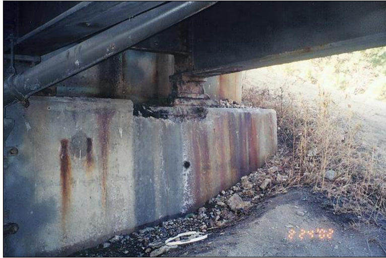
Figure 2.5.3.3-6: Large Spall on Abutment Bearing Seat – Condition State 3
