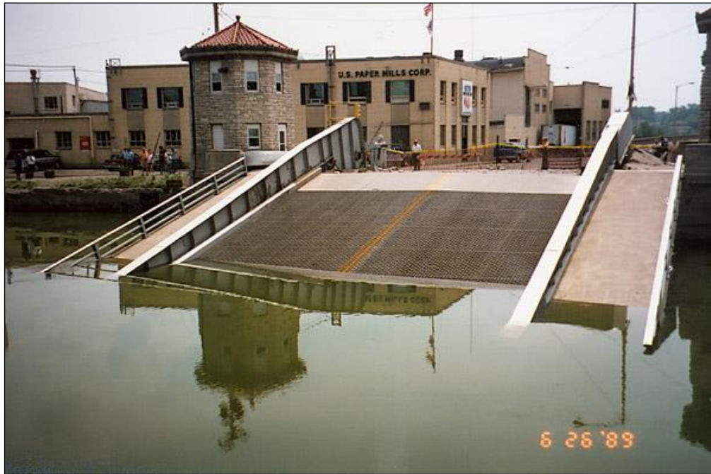
Figure 1.4.2.1-1: Failed Tayco Street Bascule Bridge, Menasha.
