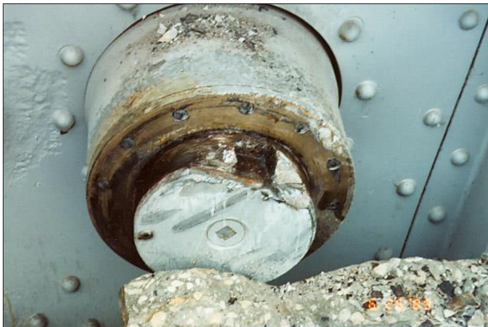
Figure 1.4.2.1-2: Failed Pin, South Bascule Span of Tayco Street Bridge.
