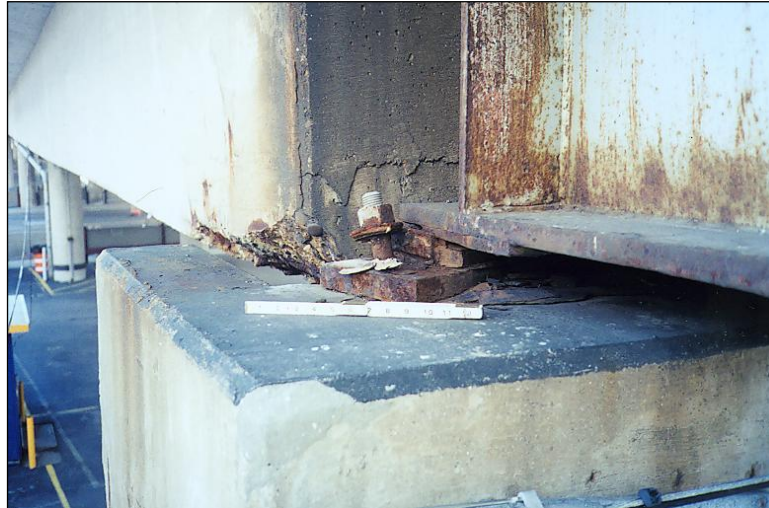
Figure 1.4.3.3-2: Failed Bearing at Pier.
