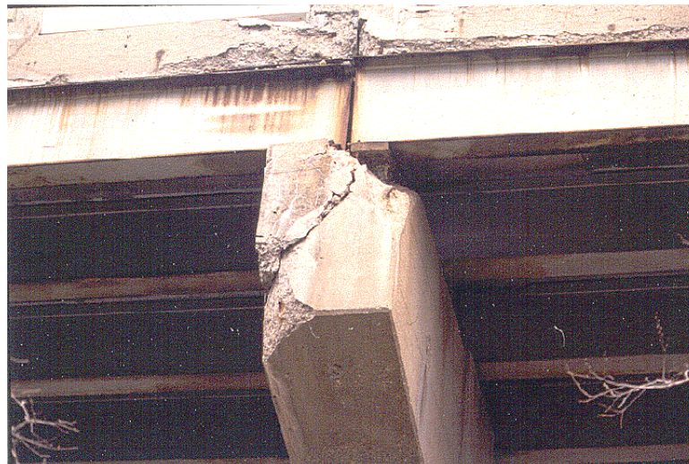
Figure 1.4.3.3-3: Damage Resulting From Failed Joint.
