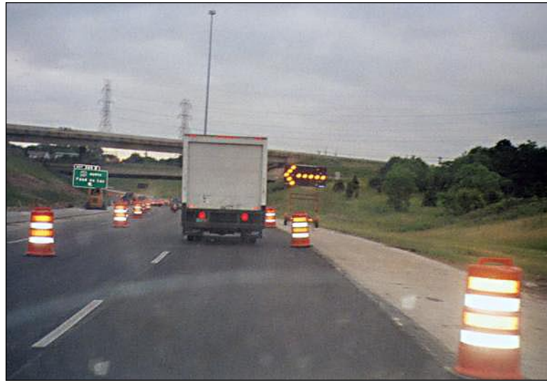
Figure 1.4.8.3-2: Directional Arrow Board and Channelizing Barrels.
