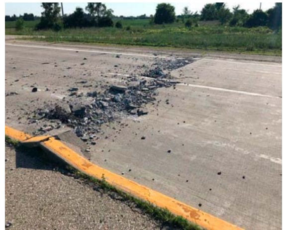
Blowup on Hwy 14 in Rock County
