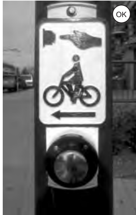
Figure 4-104: Path users need a way to trip the signal. If a loop detector is used for bicyclists, a push button for pedestrians should also be provided. Alternative means of detection (e.g., infrared) have been used for such purposes.
