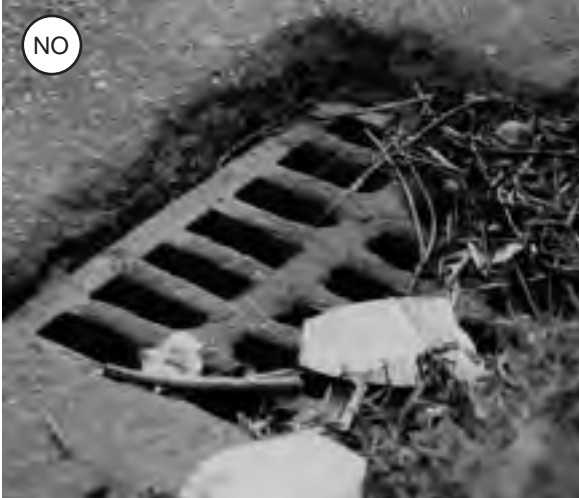
Figure 2-19: Depressed or raised grates can be hazardous, regardless of type.
