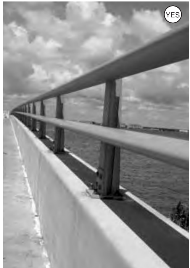
Figure 2-57: This bridge has a 54 in. railing that protects bicyclists from going over the top and into the river. Although a low-probability event, the consequences would be severe.
