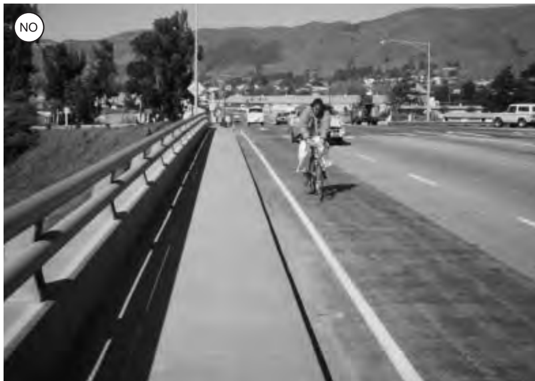
Figure 2-59: On this bridge, debris collects in the narrow striped shoulder; as a result of the surface conditions and the shoulder's width, motorists must change lanes to pass safely.
