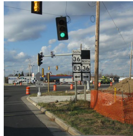
Figure 6: Temporary driveway within the functional area of an intersection
