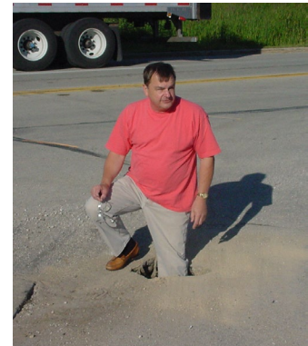
Figure 3: Improper pothole restoration
