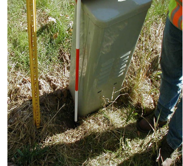
Figure 1. Pedestal too close to ROW pin.
