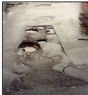
Figure 5: Both patches improperly backfilled/compacted, and not patched to nearest joint or seam
