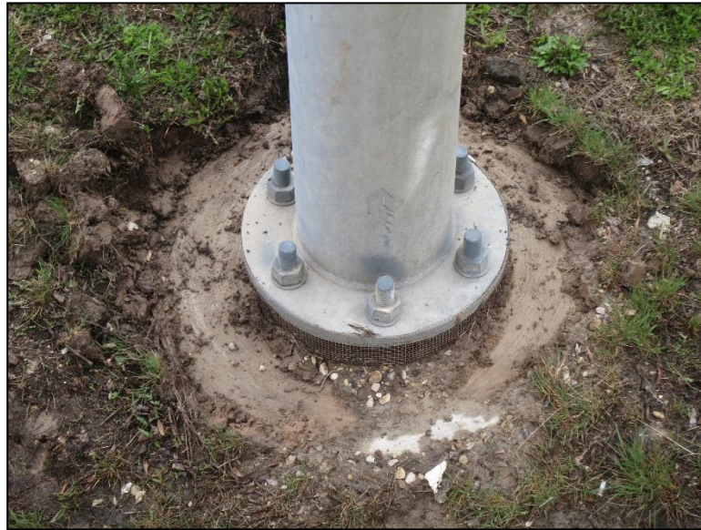
Figure 4.2.3-3: Mast Arm Foundation Initially Installed Below Grade (Condition State 2)
