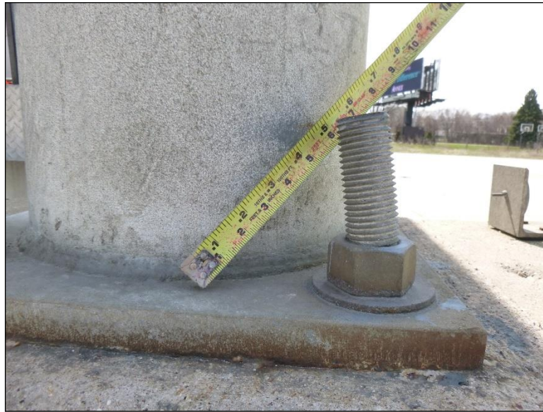
Figure 4.2.3-15: Anchor Bolt Out-of-Plumb Due to Impact (Condition State 3).
