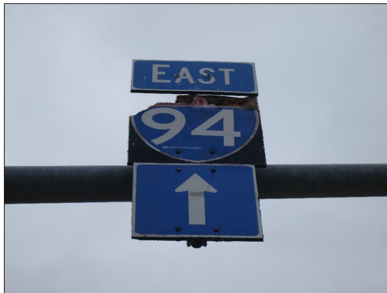
Figure 4.2.3-43: Damaged Sign Panel with Reflective Coating Missing and Fading (Condition State 3).
