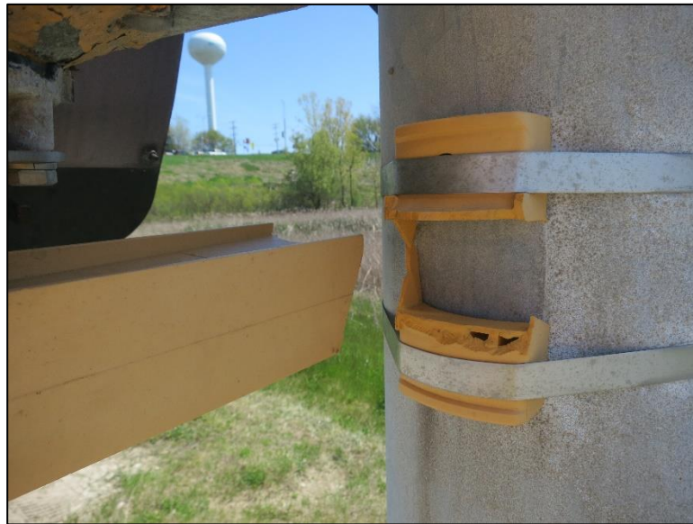
Figure 4.2.3-50: Failed Bracket to Vertical Post Connection on Monotube Structure (Condition State 4)
