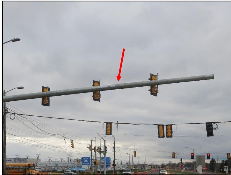
Figure 4.2.3-38: Slip Joint Extending Length of Mast Arm.
