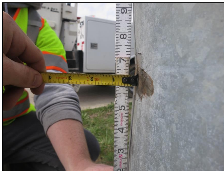
Figure 4.2.3-18: Base of Post Distorted Out of Plane Due to Impact (Condition State 3).
