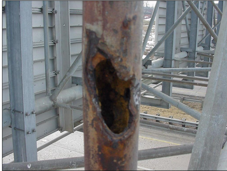
Figure 4.2.2-2: Steel Corrosion in a Vertical Member.
