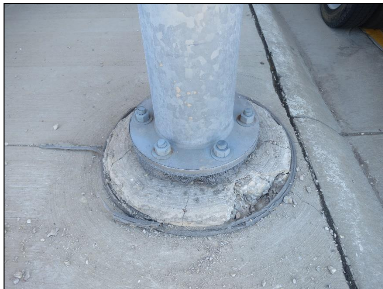
Figure 4.2.3-4: Cracked, Delaminated and Spalled Concrete Foundation (Condition State 3)
