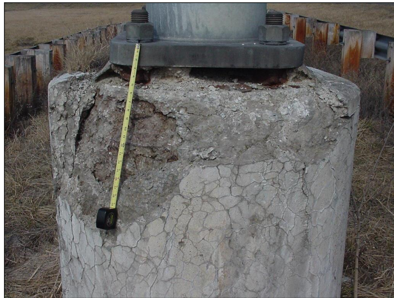
Figure 4.2.3-2: Map Cracking with Delamination and Spall on a Butterfly Foundation (Condition State 3).
