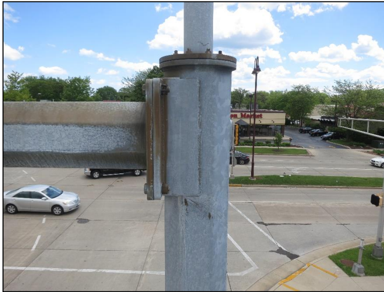
Figure 4.2.3-53: Signal Mast Arm with Luminaire Post Anchored to Top of Post. All of Luminaire is Inspected Under Element 8711.
