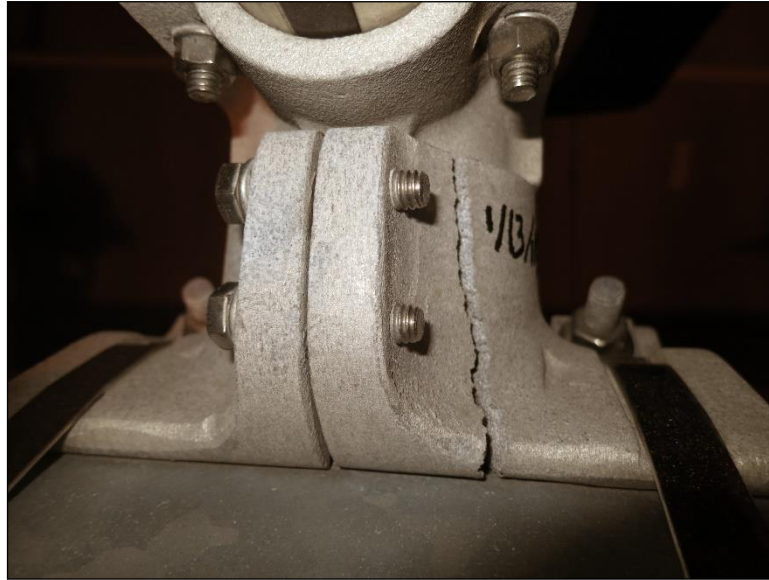
Figure 4.2.3-51: Cracked Aluminum Signal Bracket (Condition State 4)
