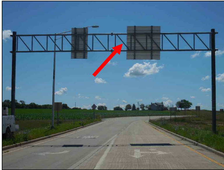
Figure 4.2.2-8: Right Truss Installed Upside Down. Truss Diagonals Should Run Down Towards Center From Upper Chord.
