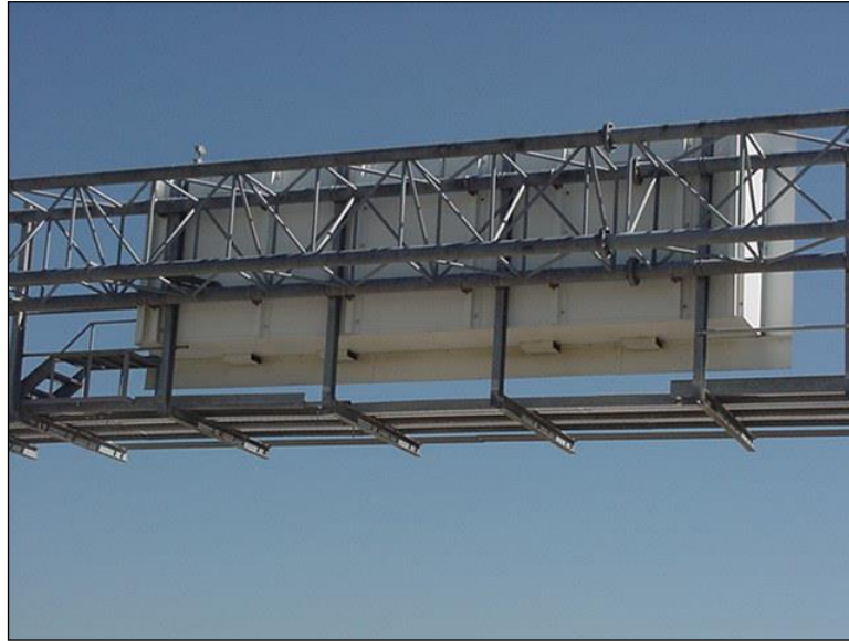
Figure 4.2.3-46: Typical Dynamic Message Sign, Rear View.
