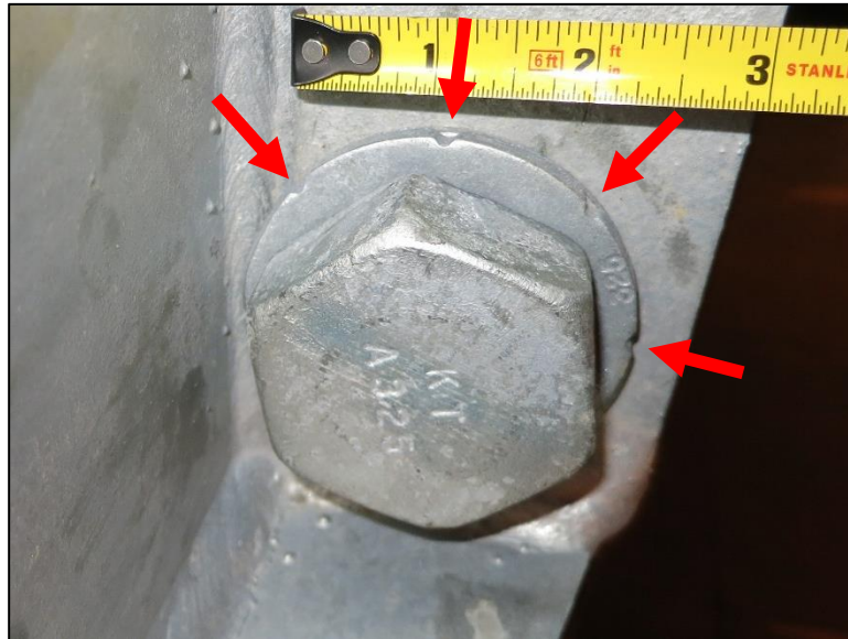
Figure 4.2.3-36: Indentations Along Edge Indicate the Component is a DTI.
