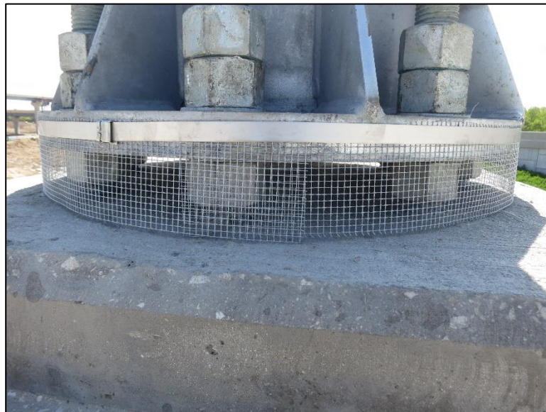
Figure 4.2.4-2: Rodent Screen Around Base Plate of Sign Structure.
