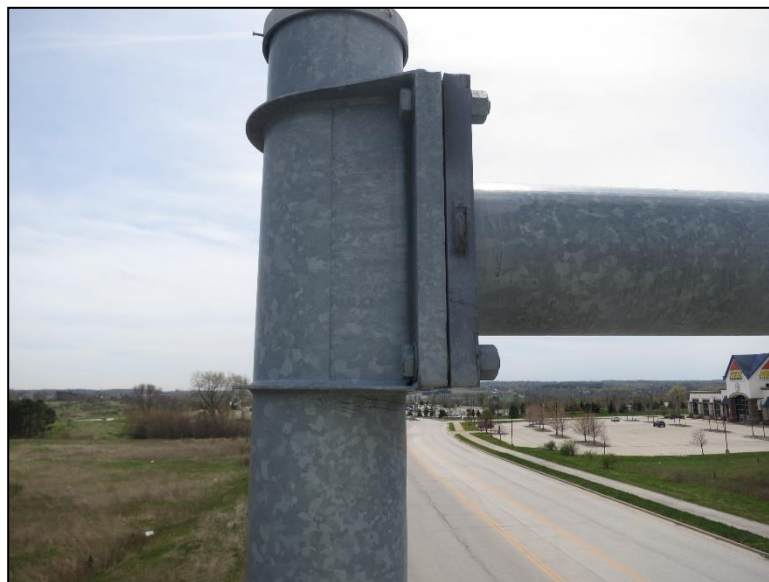
Figure 4.2.3-31: Column to Arm Connection with Horizontal Column Plates Welded to Vertical Plate. Note Washers Improperly Included Between Plates.
