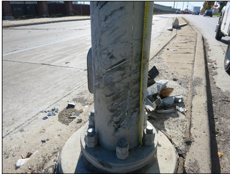
Figure 4.2.4-13: Scraped Galvanized Coating at Base of Column Due to Impact. Bare Steel Exposed in Several Locations (Condition State 3).
