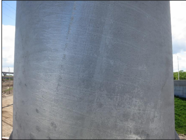
Figure 4.2.4-11: Galvanized Coating on a Steel Column of an Overhead Sign Structure. (Condition State 1).
