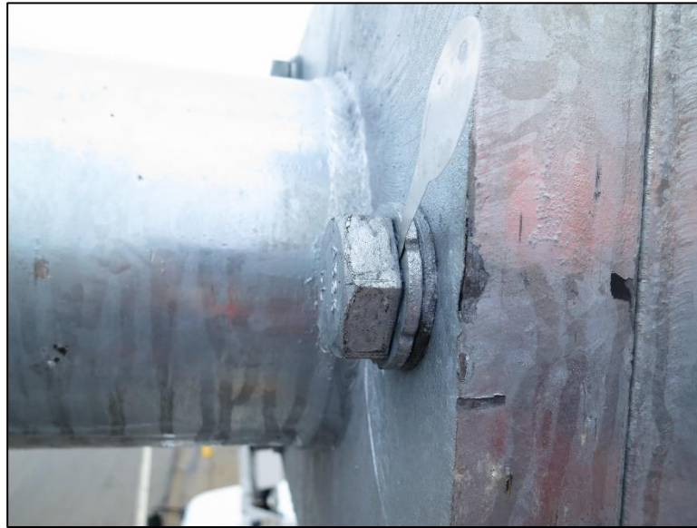
Figure 4.2.2-11: Non-Refusal of Feeler Gauge at DTI Installation.
