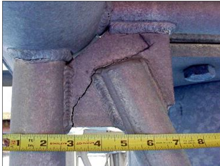
Figure 4.2.2-6: Crack through an Aluminum Gusset Plate.
