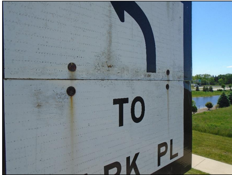
Figure 4.2.3-44: Sign Surface Cracked and Fading (Condition State 3)
