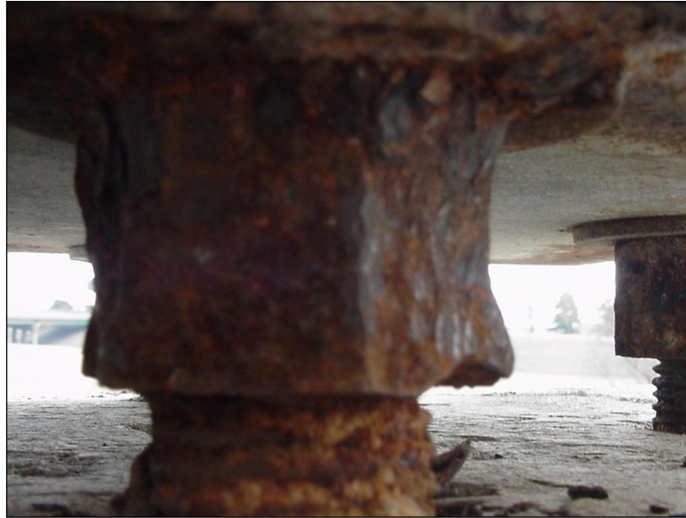
Figure 4.2.3-11: Severe Corrosion of the Leveling Nuts (Condition State 4).
