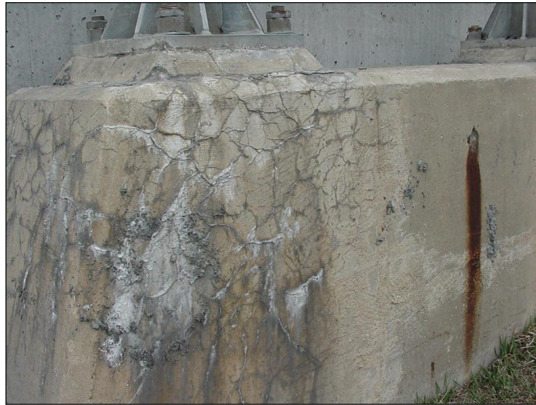
Figure 4.2.3-1: Map Cracking with Efflorescence on a Four Chord Sign Structure (Condition State 3).
