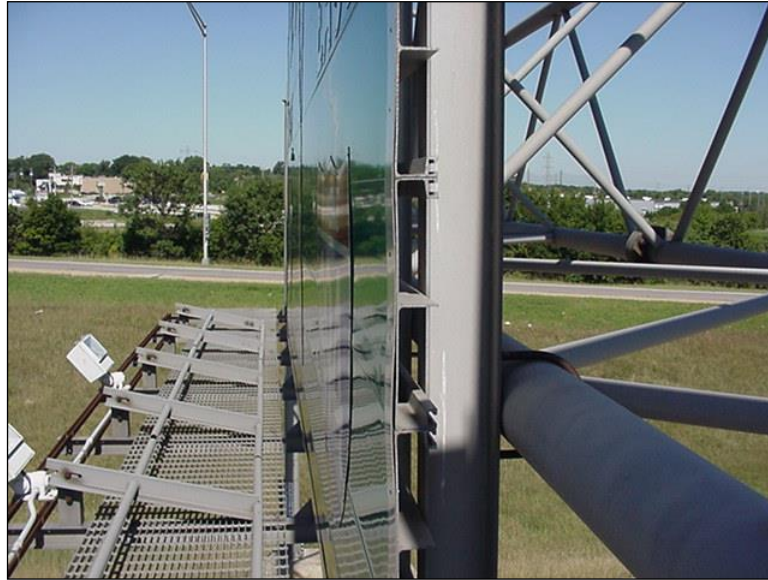
Figure 4.2.4-7: Catwalk with Handrails in Collapsed Position.
