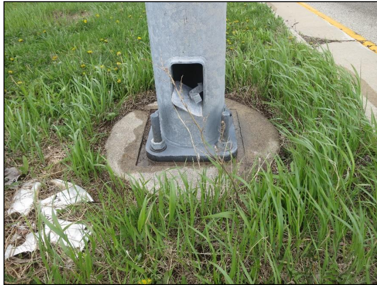
Figure 4.2.4-5: Handhole Cover Unsecured at Base of Signal Mast Arm Column (Condition State 3).
