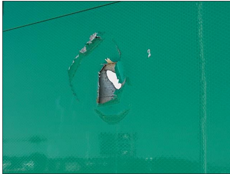
Figure 4.2.3-42: Damaged Sign Panel with Reflective Coating Beginning to Tear and Peel (Condition State 2)
