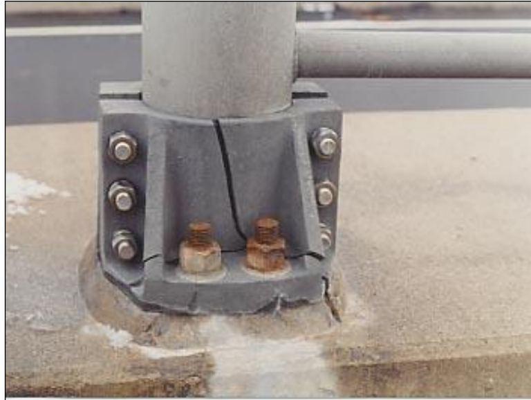
Figure 4.2.3-16: Failed Aluminum Base Casting Clamp Initiated by Over-tightening the Stainless Steel Horizontal Column Bolts.
