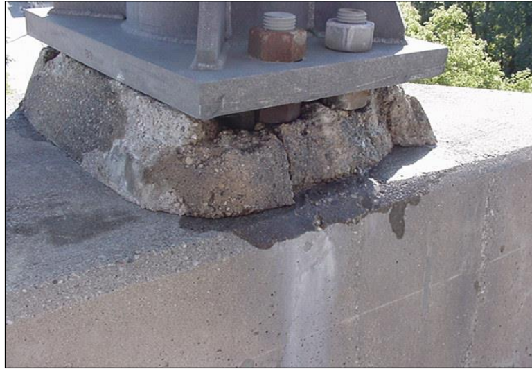
Figure 4.2.3-7: Deteriorated Grout Pad (Condition State 3).
