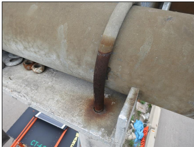
Figure 4.2.3-30: Corroded U-Bolt Connection Securing Horizontal Sign Support Member to the Post of a Butterfly Sign Structure (Condition State 2).
