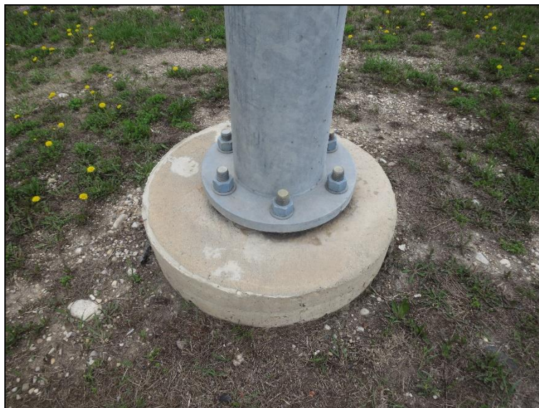
Figure 4.2.3-6: Anchor Rods Installed Offset from Center Foundation (Condition State 2 if Verified by Engineer within Report).
