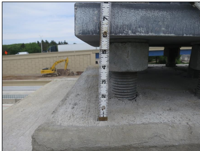
Figure 4.2.3-14: Excessive Anchor Rod Stand-Off from Foundation (Condition State 3).
