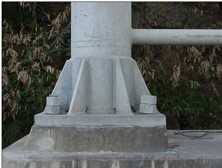
Figure 4.2.3-10: Anchor Bolt Installed Out-of-Plumb Greater than 1:40 (Condition State 3).
