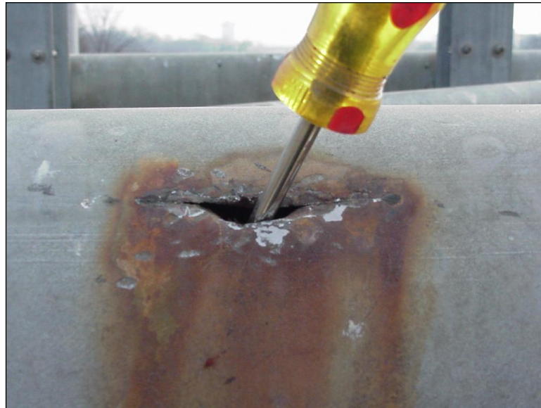
Figure 4.2.2-4: Split Associated with Corrosion in a Horizontal Chord Member.
