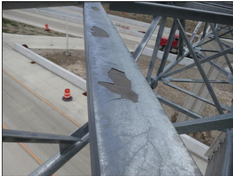
Figure 4.2.4-12: Cracked, Chipped and Peeling Galvanized Protective Coating on a Four-Chord Upper Diagonal Member (Condition State 3)
