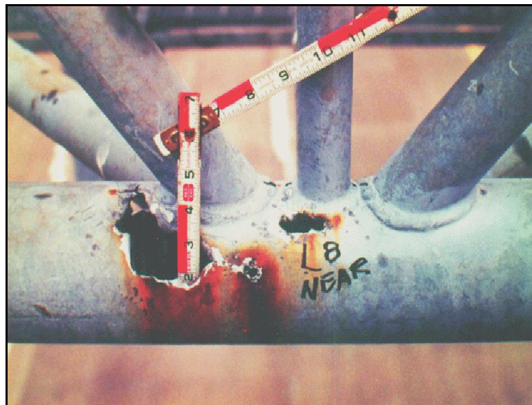
Figure 4.2.2-3: Corrosion in a Horizontal Steel Chord Member.
