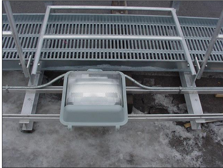
Figure 4.2.4-3: Typical Sign Structure Luminaire.
