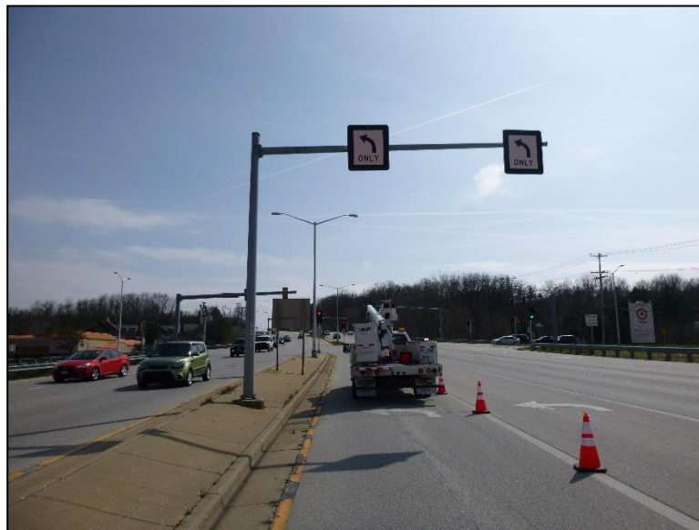
Figure 4.2.1-9: Typical Mast Arm Sign Support.
