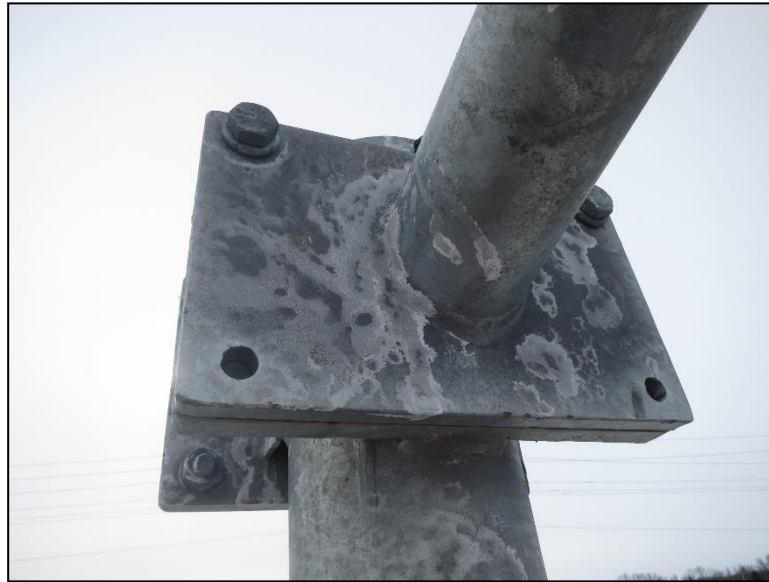
Figure 4.2.3-34: Missing Lower Connection Bolts of a 4 Bolt Connection (Condition State 4).
