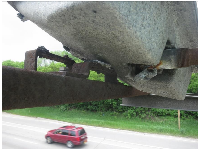
Figure 4.2.4-4: Failed Connections of a Luminaire to U-Bracket on a Butterfly Sign Structure (Condition State 4)
