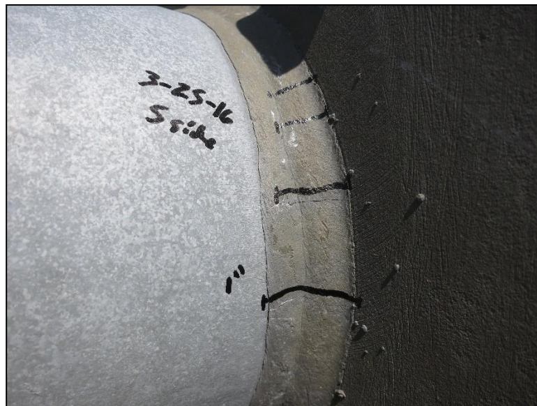
Figure 4.2.3-35: Transverse Weld Cracks Along Circumferential Socket Weld of Mast Arm to Vertical Plate Connection (Condition State 3)
