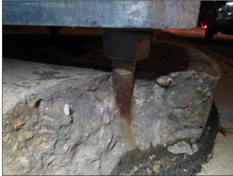
Figure 4.2.3-5: Foundation Spall Exposing Anchor Rod (Condition State 3).
