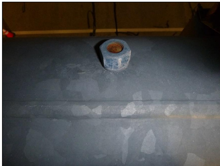
Figure 4.2.3-39: Slip Joint Through Bolt Nut Not Fully Engaged.
