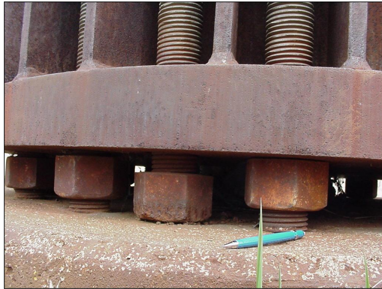
Figure 4.2.3-13: Leveling Nuts Not Fully In Contact with the Base Plate (Condition State 4).
