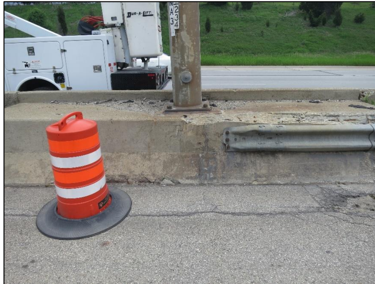
Figure 4.2.4-9: Deteriorated Barrier Wall with Approach Guardrail Protecting the Foundation of a Butterfly Sign Structure (CS 2)
