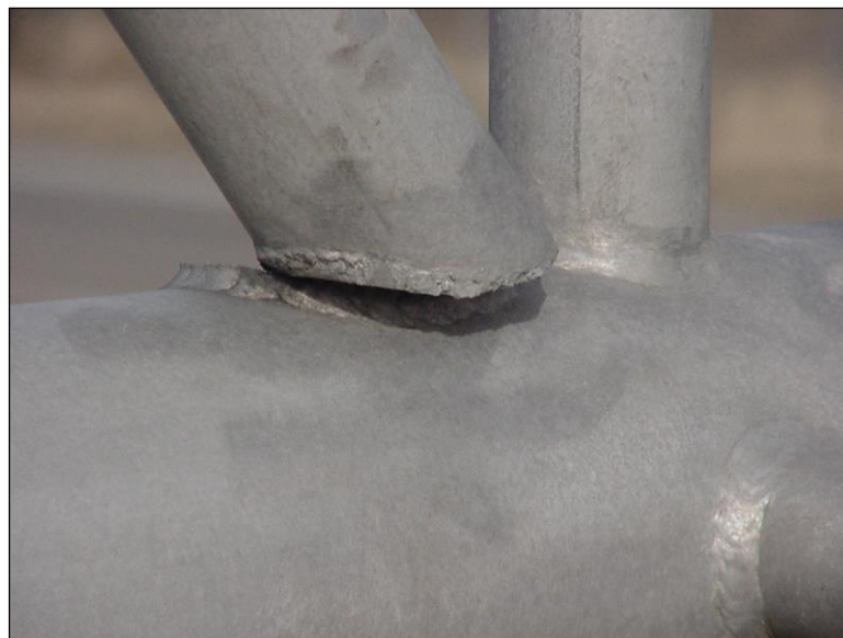
Figure 4.2.2-5: Broken Weld at an Aluminum Diagonal Member.
