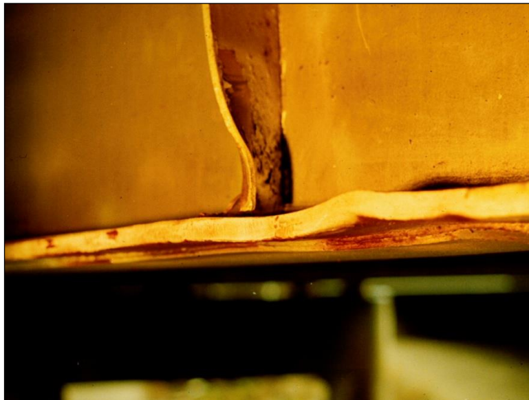
Figure 2.1.4.2-8: Girder Bottom Flange Impact Damage.
