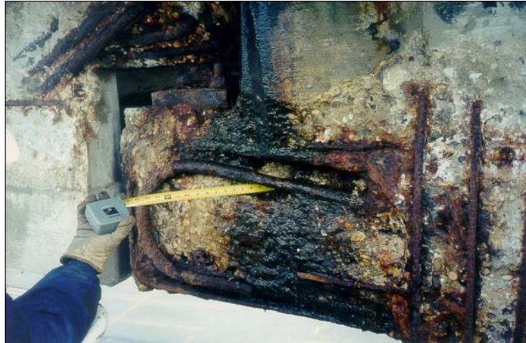
Figure 2.1.4.1-7: Reinforcing Steel Corrosion.
