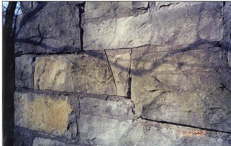
Figure 2.1.4.4-2: Split Masonry Unit with Failing Mortar Joints.
