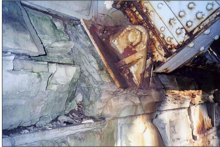
Figure 2.1.4.4-1: Masonry Deterioration/Spalls at an Arch Bearing.
