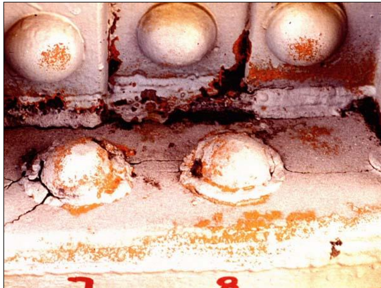
Figure 2.1.4.4-4: Fatigue Cracks on a Steel Casting.
