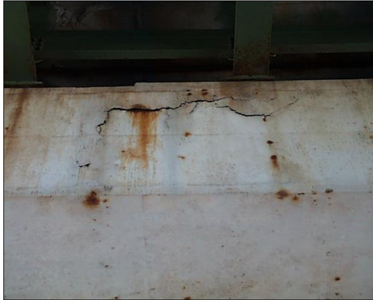
Figure 2.1.4.1-5: Delaminations on Concrete Pier.
