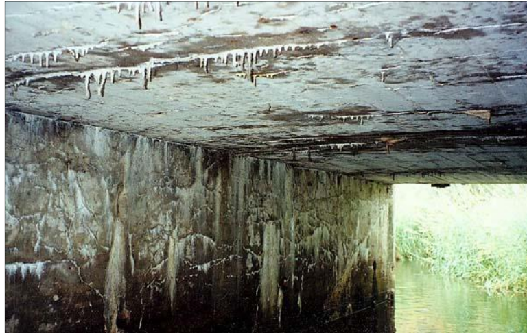
Figure 2.1.4.1-8: Heavy Efflorescence on an Abutment and Slab.
