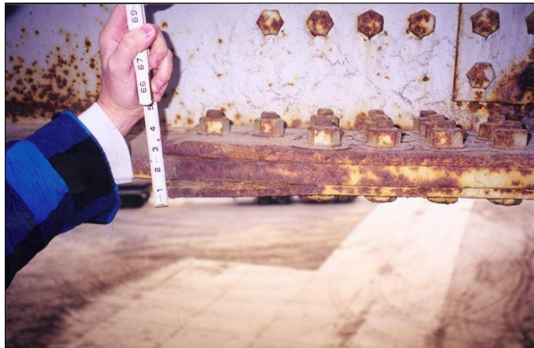
Figure 2.1.4.2-7: Pack Rust Prying Apart Flange Splice Plates.
