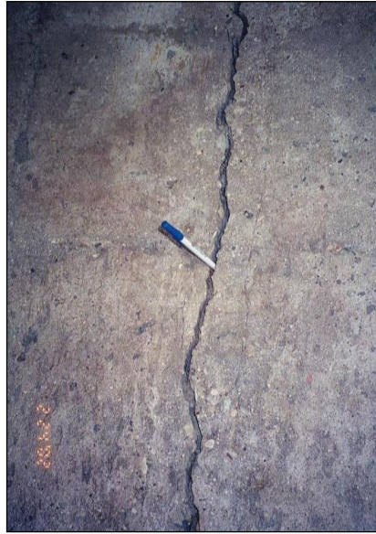
Figure 2.1.4.1-3: Wide Vertical Crack in an Abutment.
