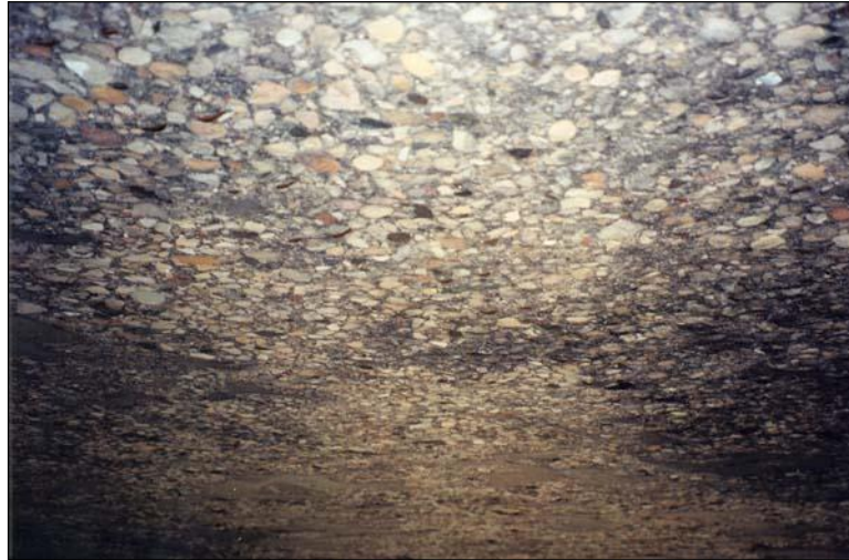
Figure 2.1.4.1-9: Scaling on the Underside of a Concrete Box Girder Due to Fire.
