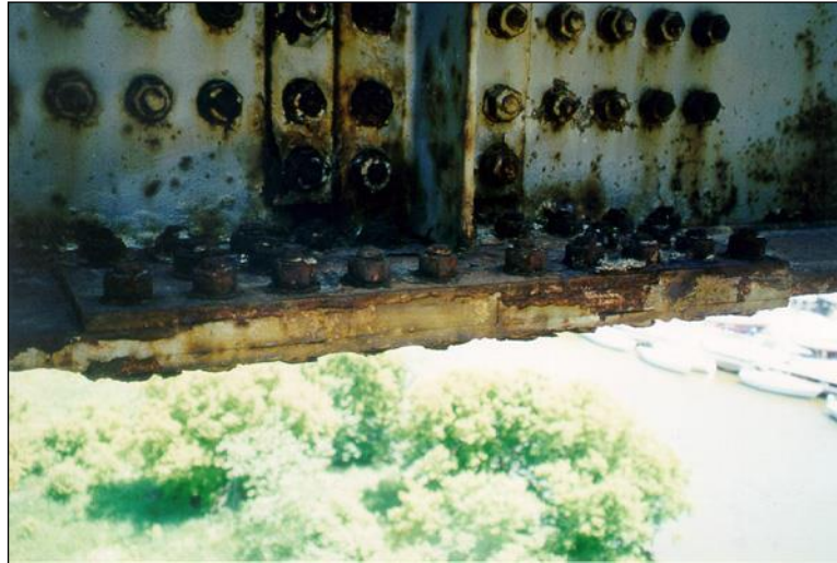
Figure 2.1.4.2-5: Steel Corrosion at Girder Splice.
