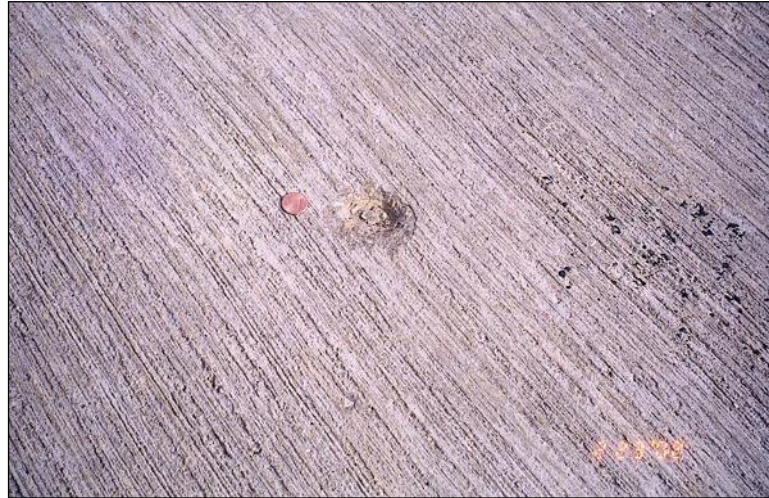
Figure 2.1.4.1-10: Pop-out on Concrete Deck.
