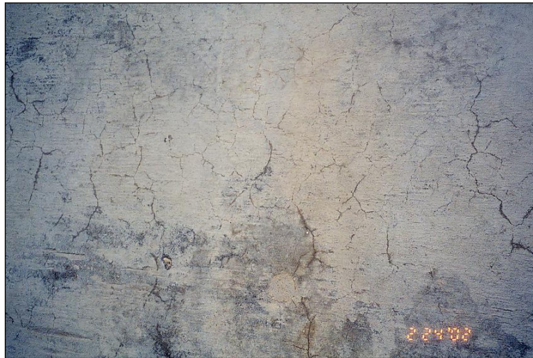
Figure 2.1.4.1-1: Map Cracking in Reinforced Concrete.
