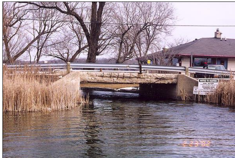
Figure 2.1.5.1-1: Heavily Deteriorated Single Span Concrete Slab.
