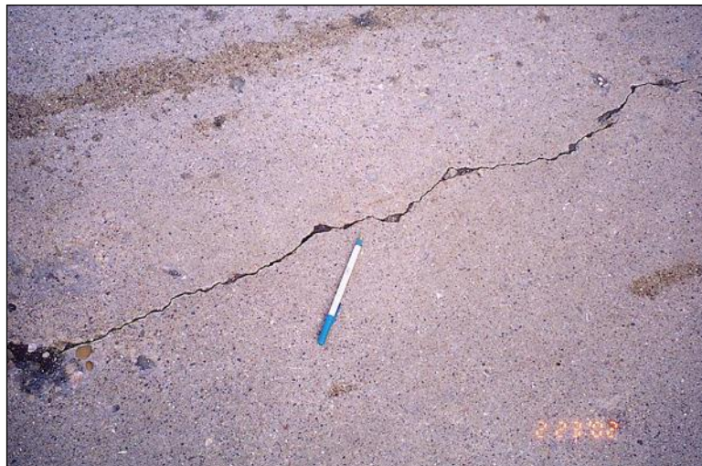
Figure 2.1.4.1-2: Moderate Longitudinal Crack in a Concrete Deck.
