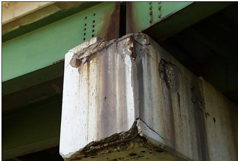
Figure 2.1.4.1-6: Spalled Concrete on Pier Cap.
