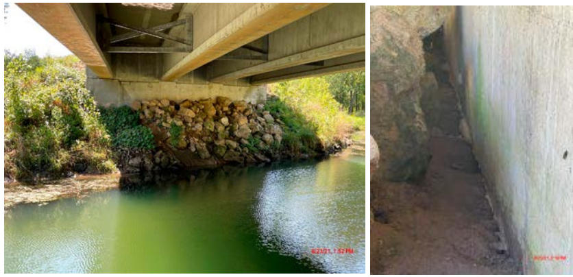
Photos of an abutment and a close-up of erosion along the abutment
