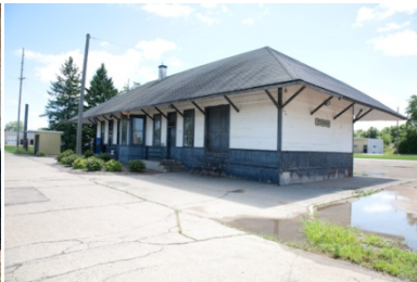
View of building from platform. Note cracked pavement and drainage problem.
