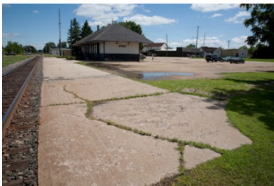
Platform. No tactile edge, below top-of-rail, and cracked pavement
