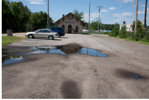
Gravel parking with drainage problems
