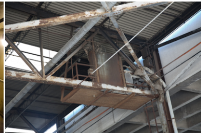
Deteriorated girders and roof
