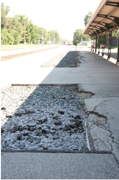
Area between platform and building. Note ballast and gravel areas, and cracked pavement.
