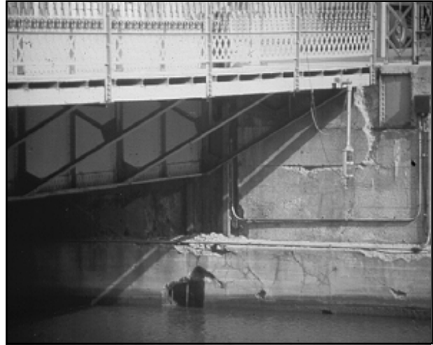
Figure 14. When the supporting foundation deteriorates, complete bridge replacement is necessary.
