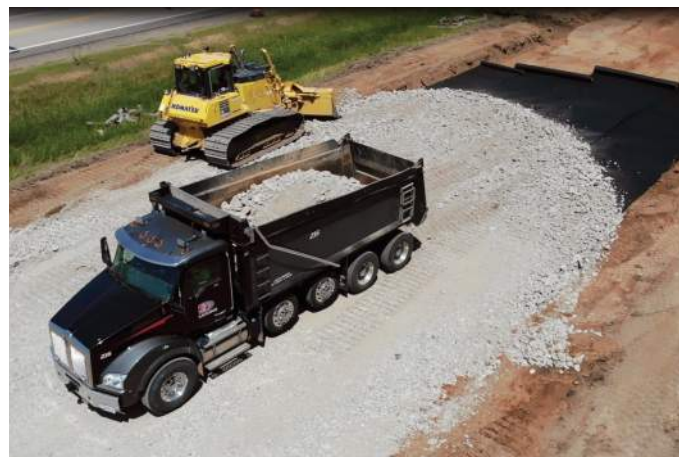
DBE trucking firm CT Enterprises of Sand Creek, LLC and geotextile fabric supplied by DBE Heider & Bott Company.
