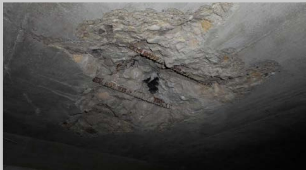
Exposed rebar in underside of slab
