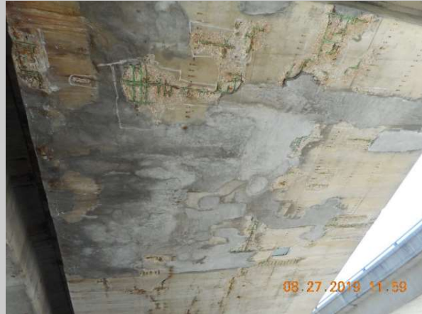
Deteriorating concrete box girder
